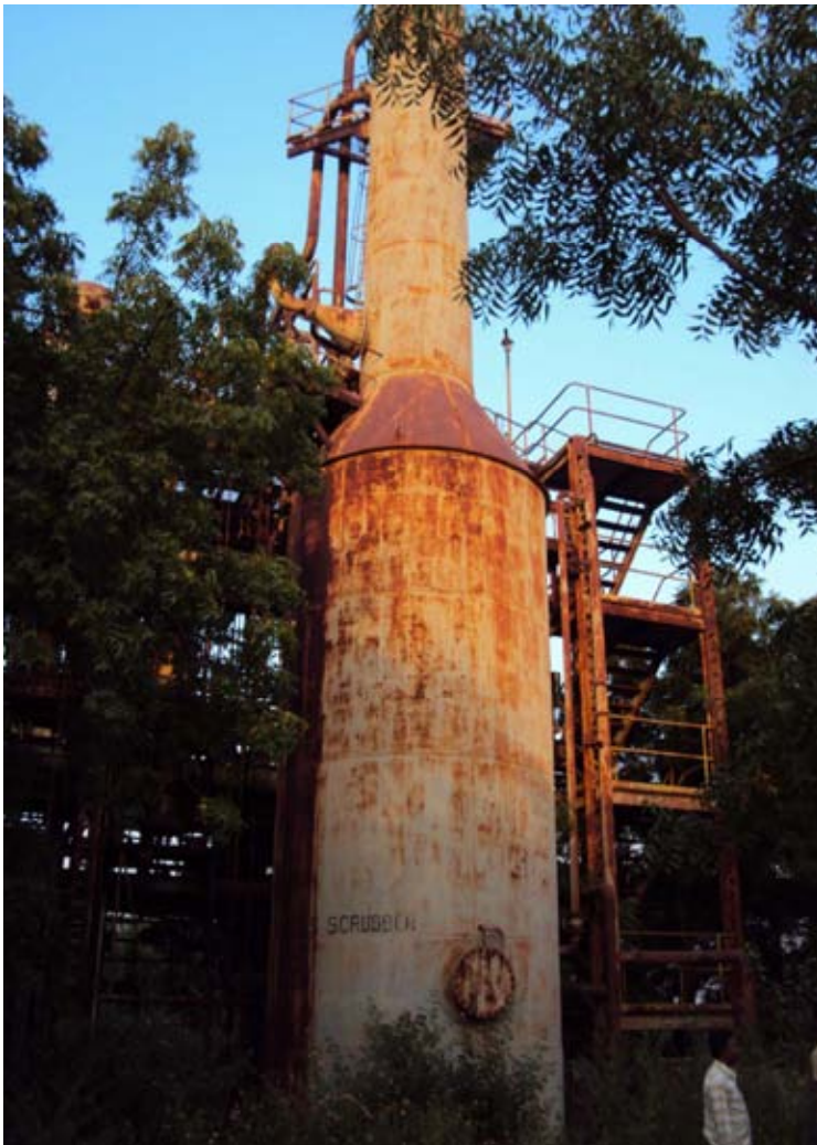
Vent Gas Scrubber at UCIL
