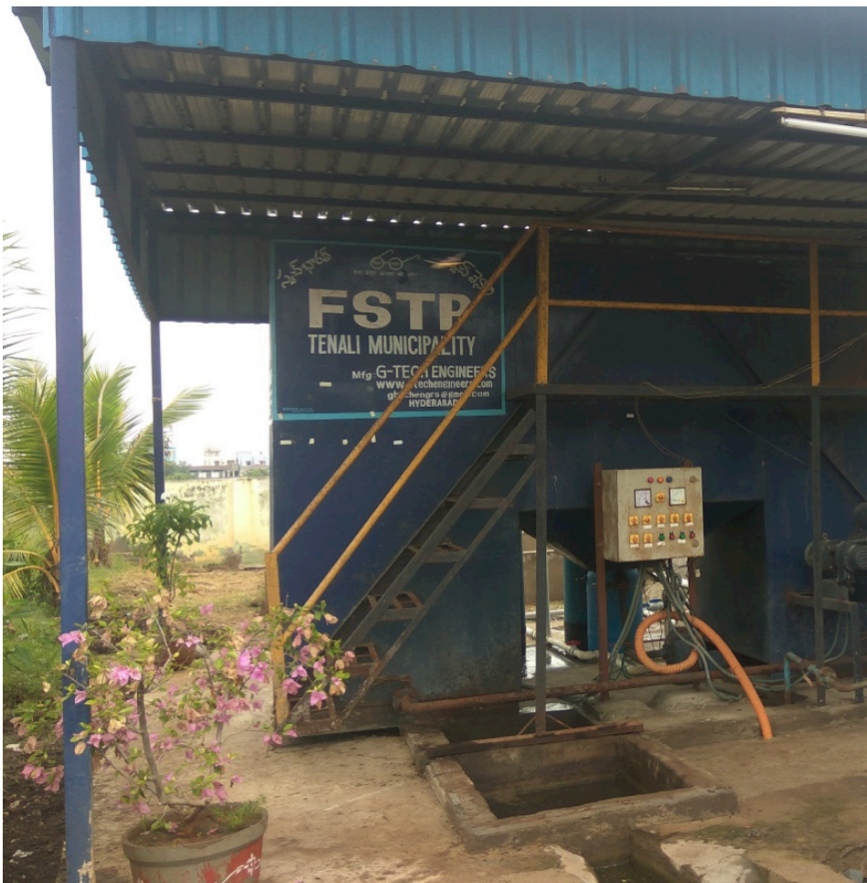
MBBR technology for the treatment of faecal sludge at the Tenali FSTP
