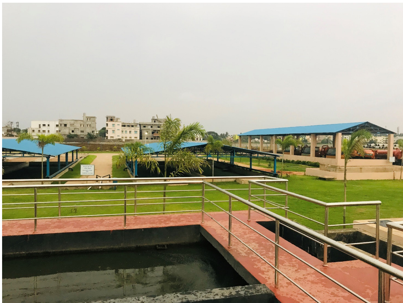
Faecal sludge settling–thickening tanks and dried-sludge storage sheds at the Bhubaneswar FSTP
