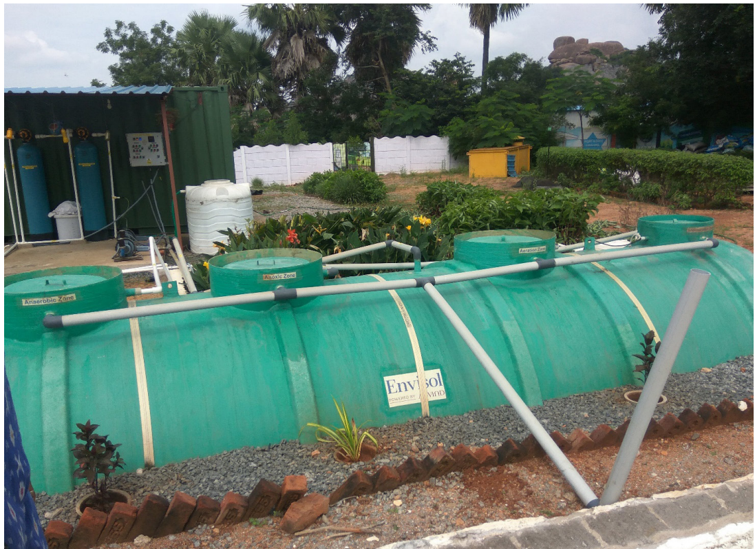
Package STP for the treatment of leachate at the Warangal FSTP
