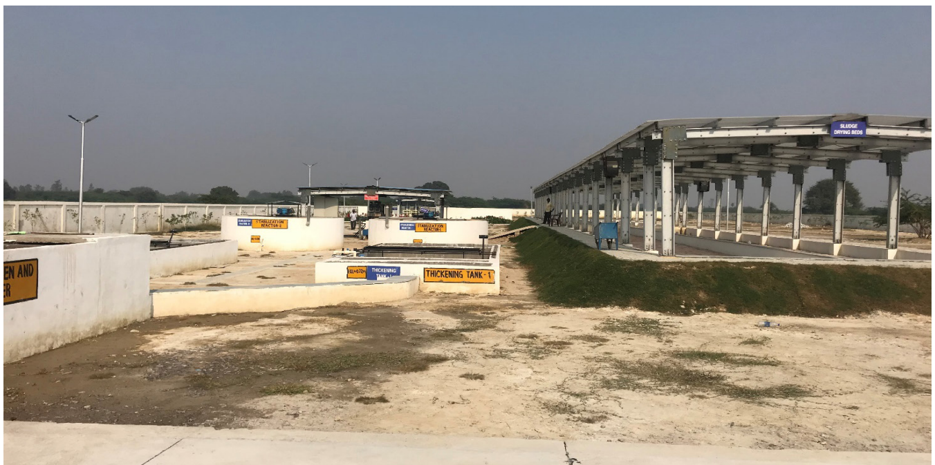
Unplanted sludge drying bed and sludge thickening tank at the Unnao FSTP
