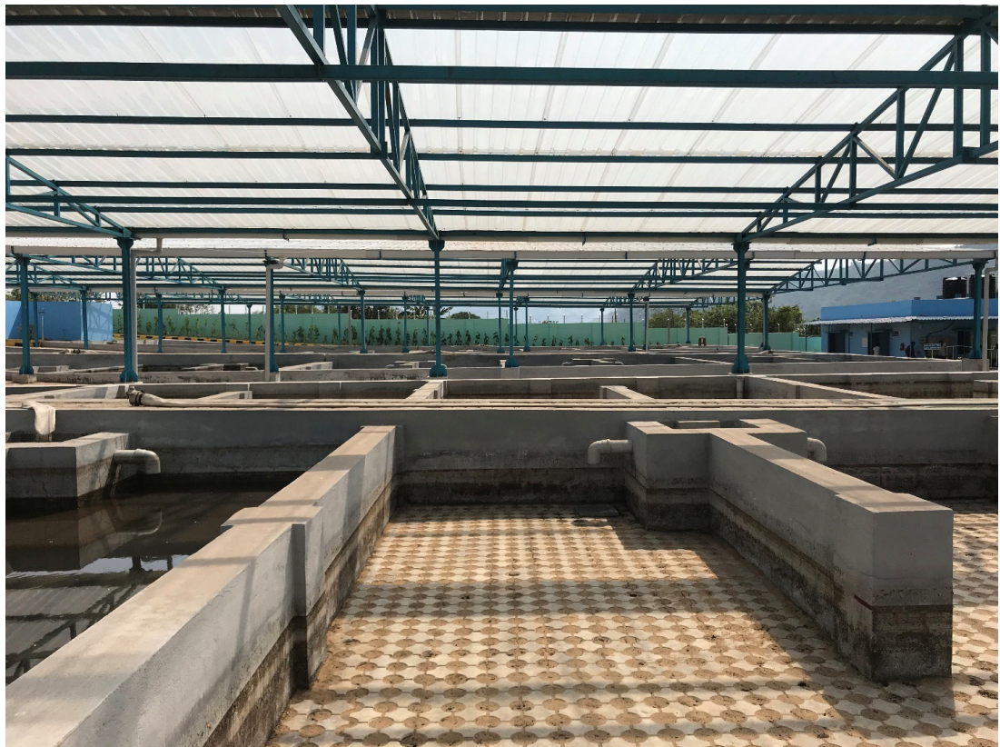
Unplanted sludge drying bed at the Dhenkanal FSTP
