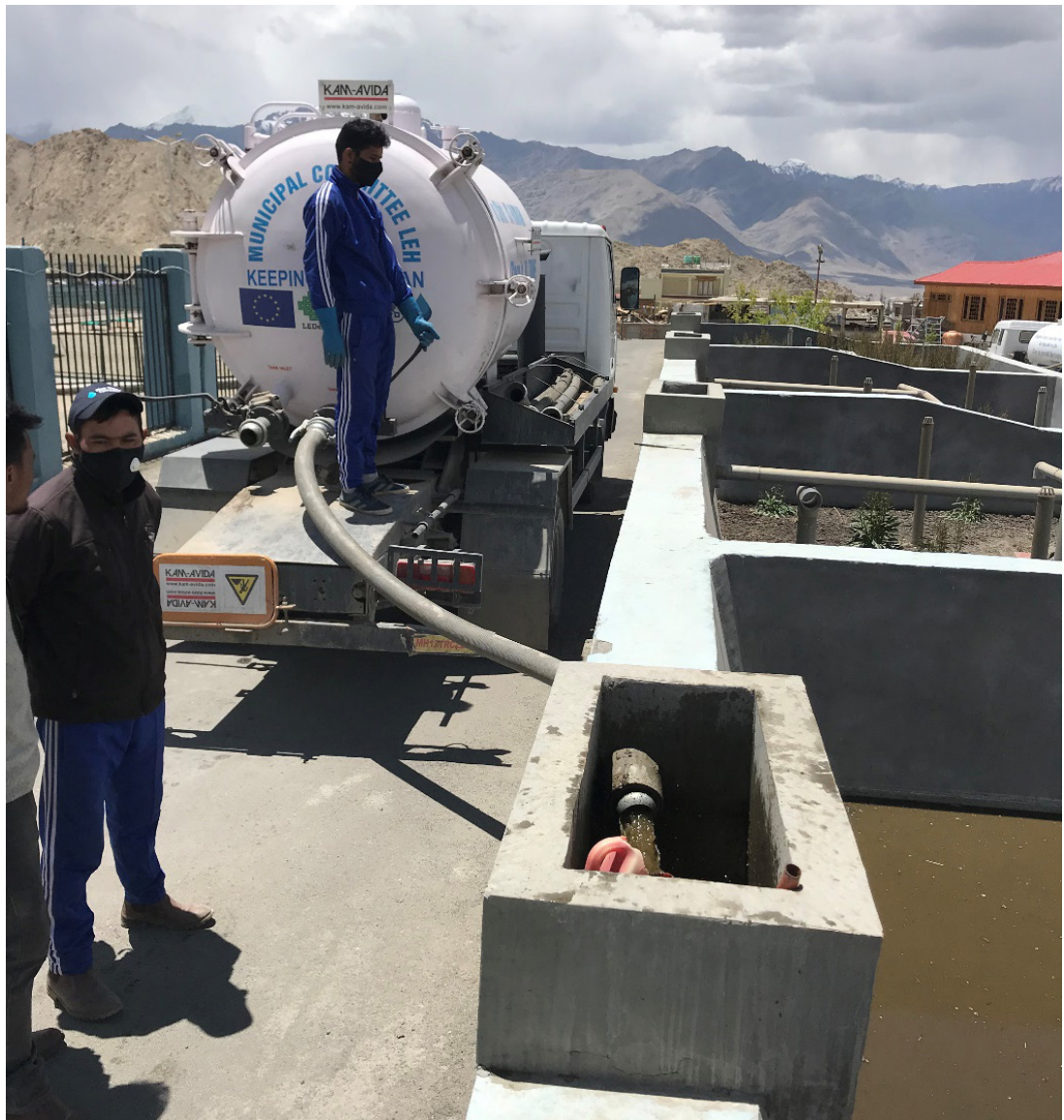
Discharging faecal sludge to planted sludge drying bed at the Leh FSTP
