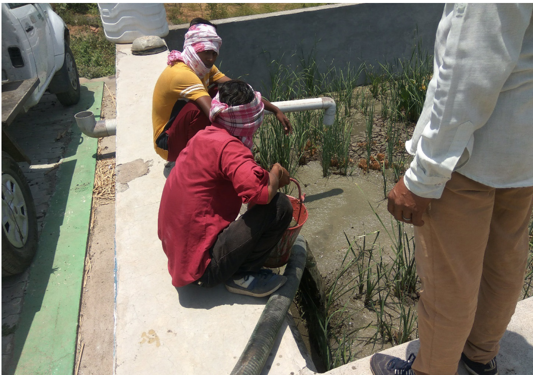
Planted sludge drying bed at the Jhansi FSTP
