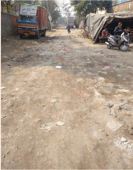
Image 18: Bad condition of the roads in industrial areas
