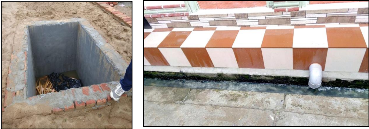
Figure 8: Fully lined tank under construction and effluent overflowing through elbow (Source: draft CSP, 2019)
