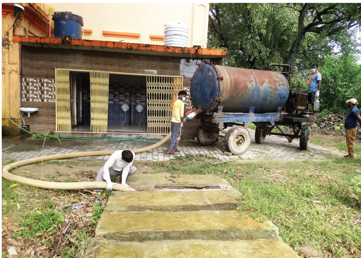
Mechanical emptying of containment system, Pilibhit
