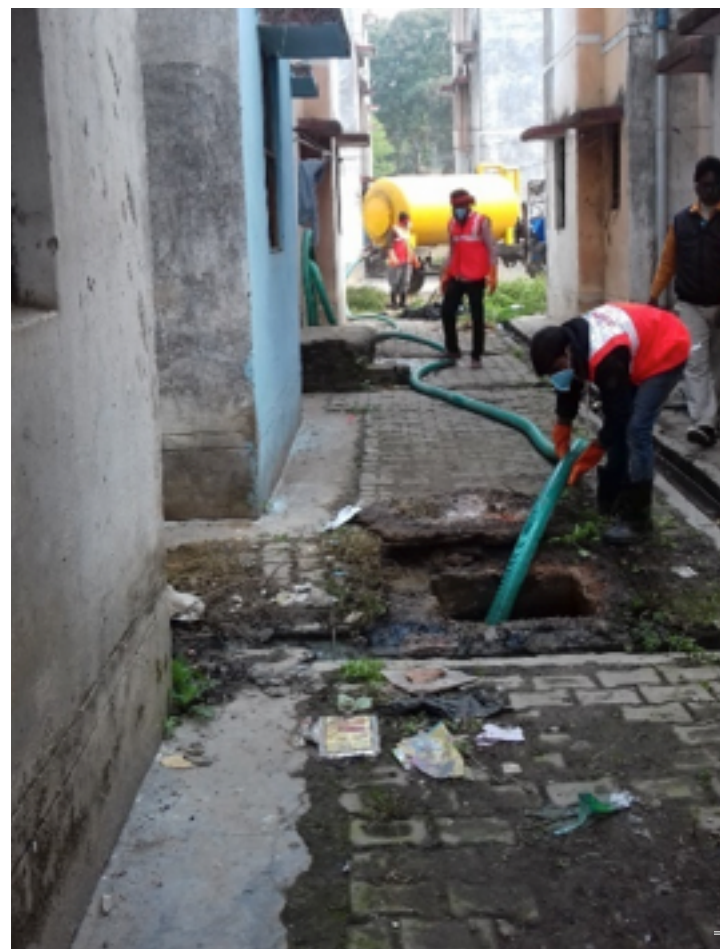
Mechanical emptying of faecal sludge by government operated tractor mounted vacuum tanker, Chunar
