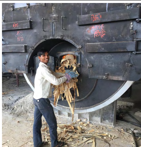
Image 5: Wood fired steam boiler, required for steam generation which is used for pressing of veneers
