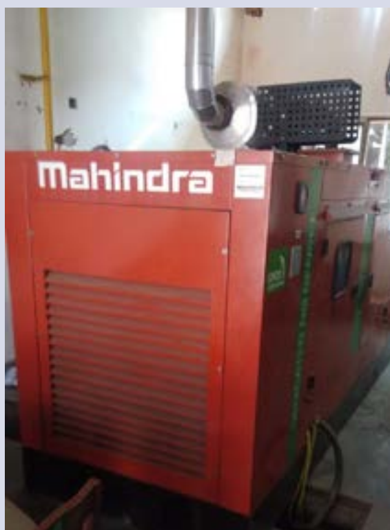
Natural gas generator installed at Hamdard Laboratories
