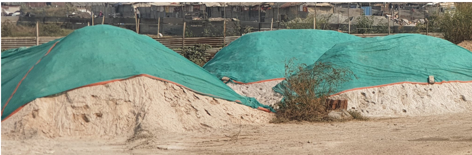
Mitigation measures such as covering materials can be adopted to suppress dispersal of dust produced due to construction activities
