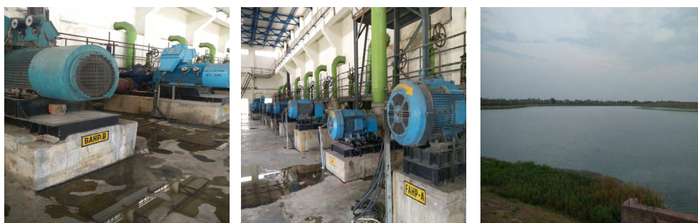
Bottom ash handling pumps
