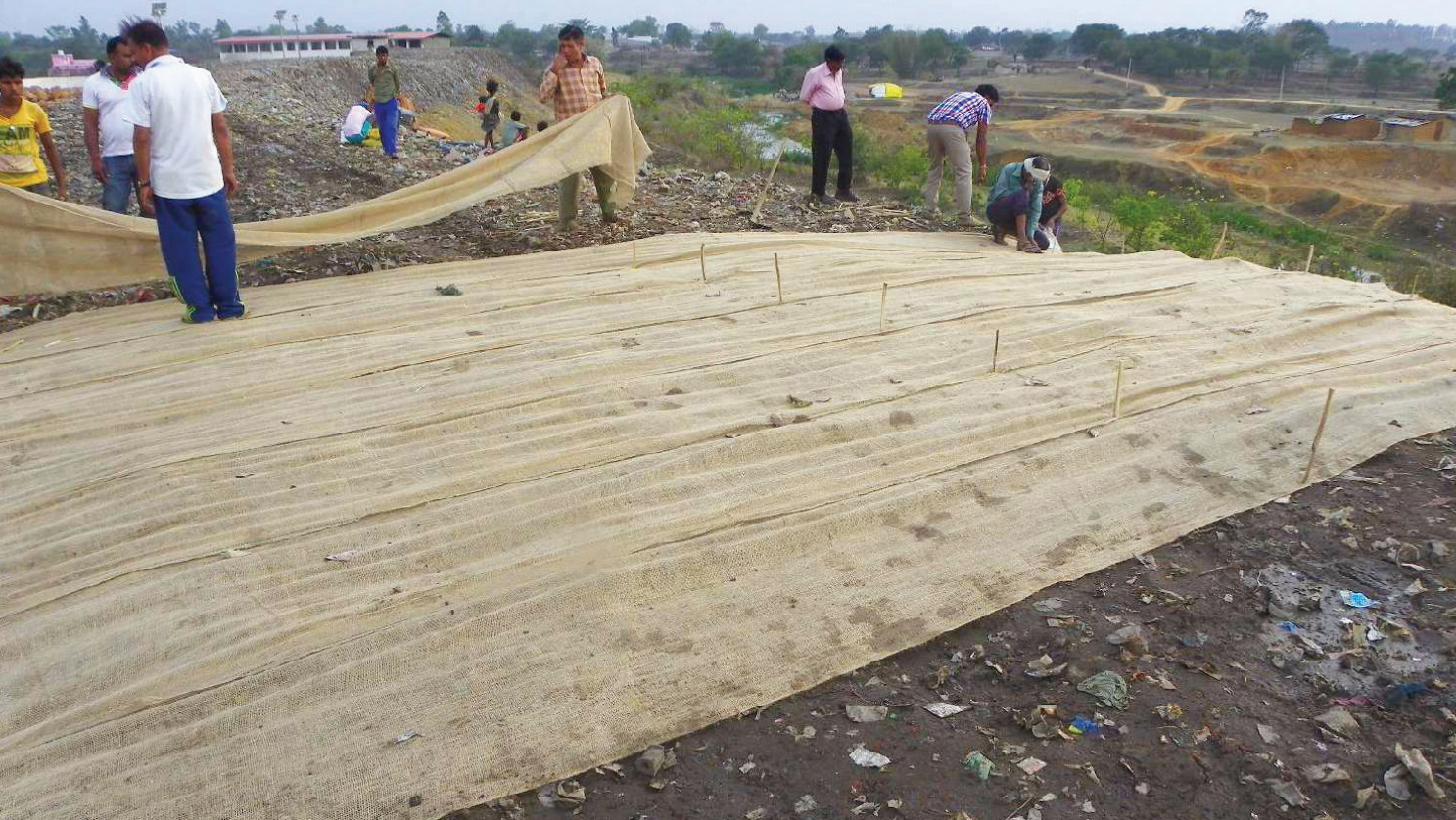
Legacy waste treatment: Jute capping, after which the entire waste surface is covered with capping materials like leaf mulch/organic manure/compost for two inches for cultivating local grass/ragi to bind the soil on the surface
