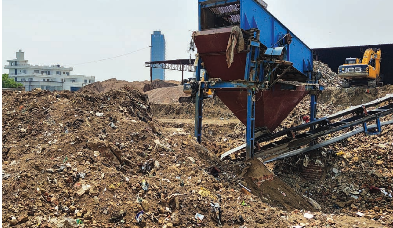
A crusher to process C&D waste at the Basai plant
