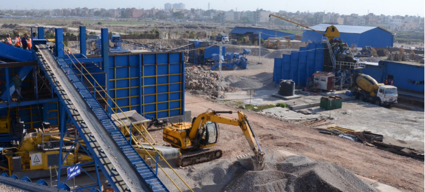
C&D waste processing plant, Burari
