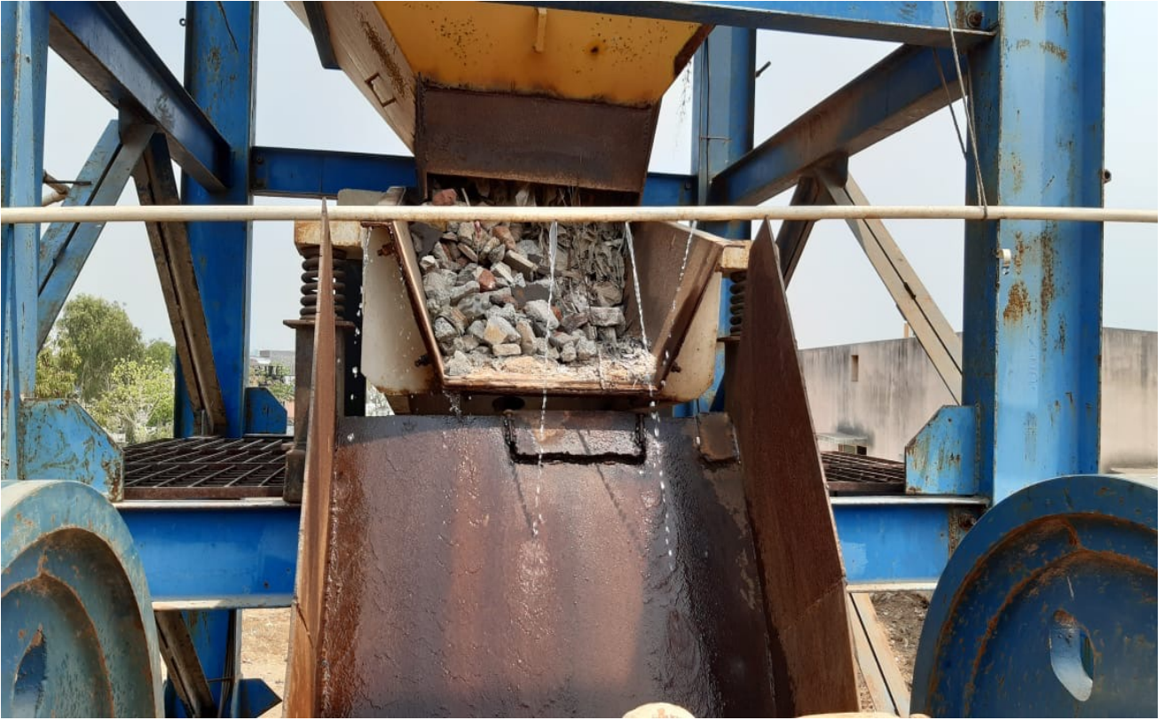
C&D waste processing facilities in Vijayawada
