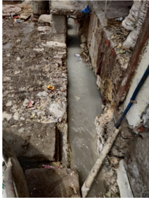
Petha waste is found dumped in drains
