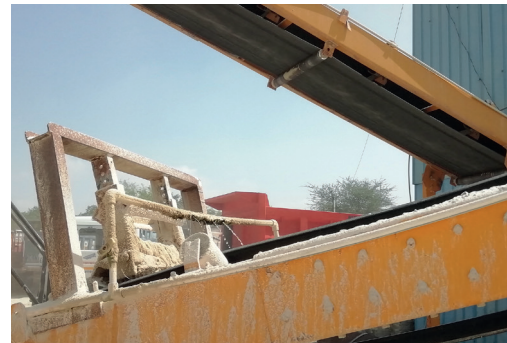
Working but inefficient water sprinkler
