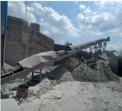
Halfhearted attempted in covering conveyor belt
