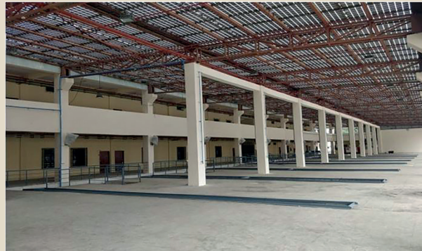
Inspection pit covered by solar panel
