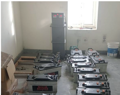
Image 32: Wrong practice Battery is placed directly on ground while charging
