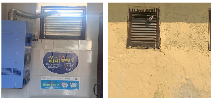
Decentralized incinerator installed in a public toilet in a park in Gurugram
