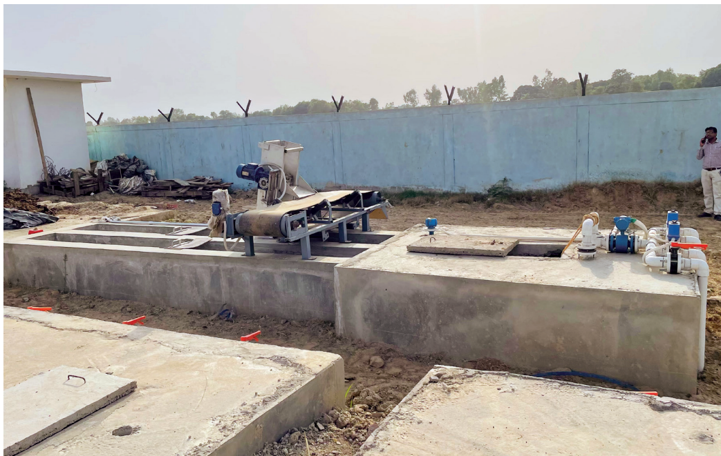
Screening unit at FSTP Pilibhit
