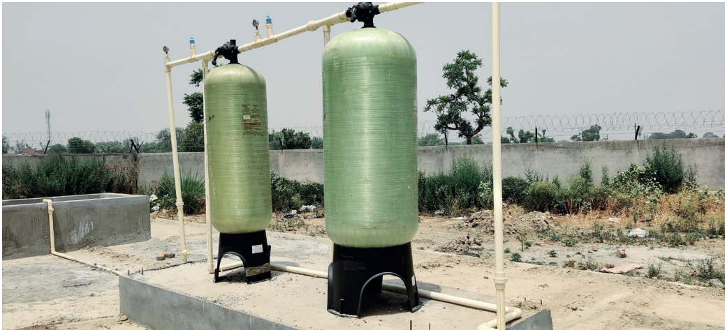
Pressurised sand and activated carbon filter for advance treatment at Hathras
