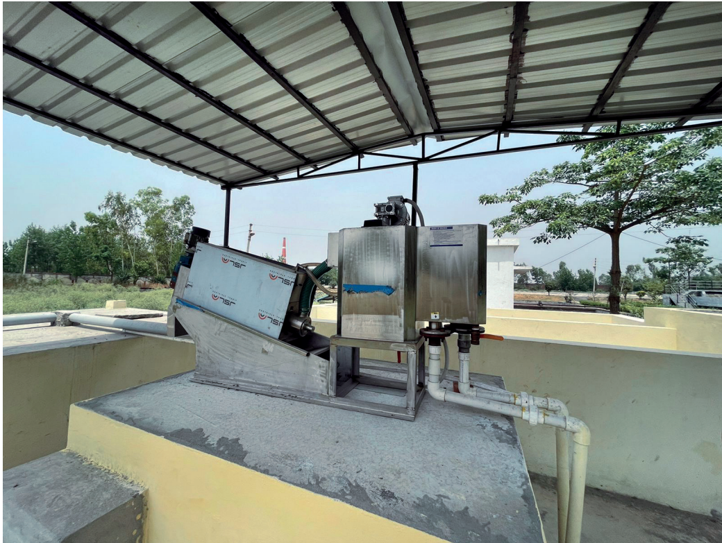
Mechanical de-watering unit at co-treatment plant, Mathura
