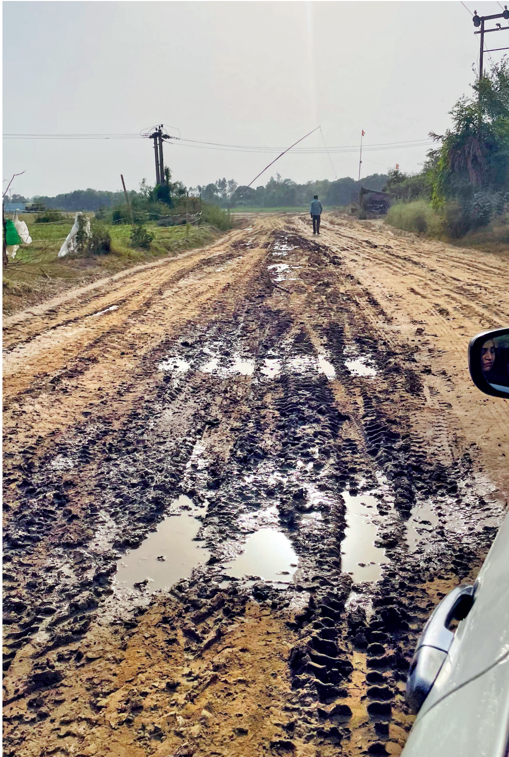
Improper approach road to FSTP in Pilibhit
