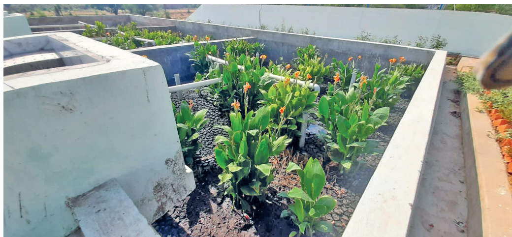
Planted drying bed technology at Chunar
