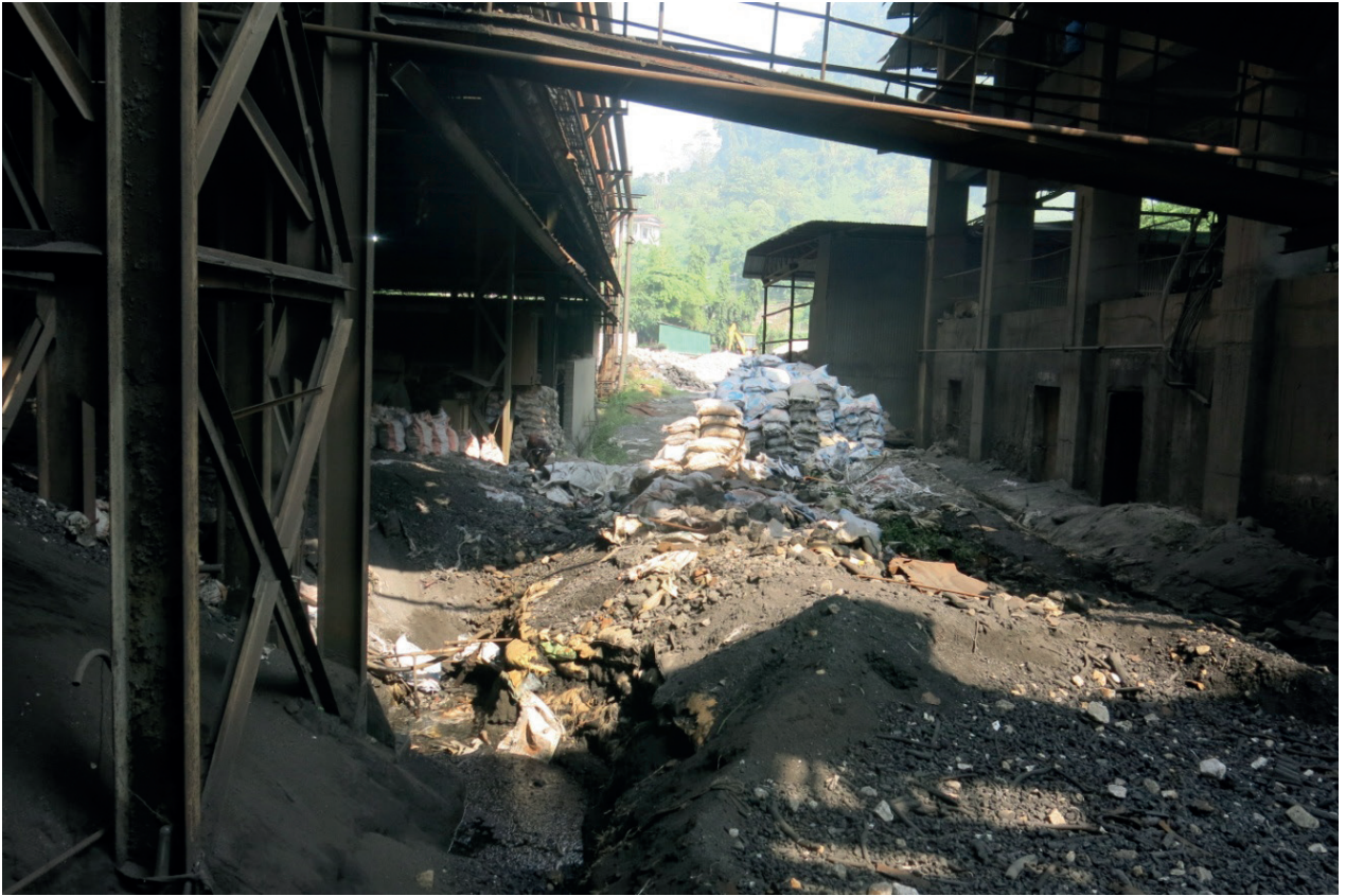
Figure 26: Access to stack and gas cleaning plant blocked
