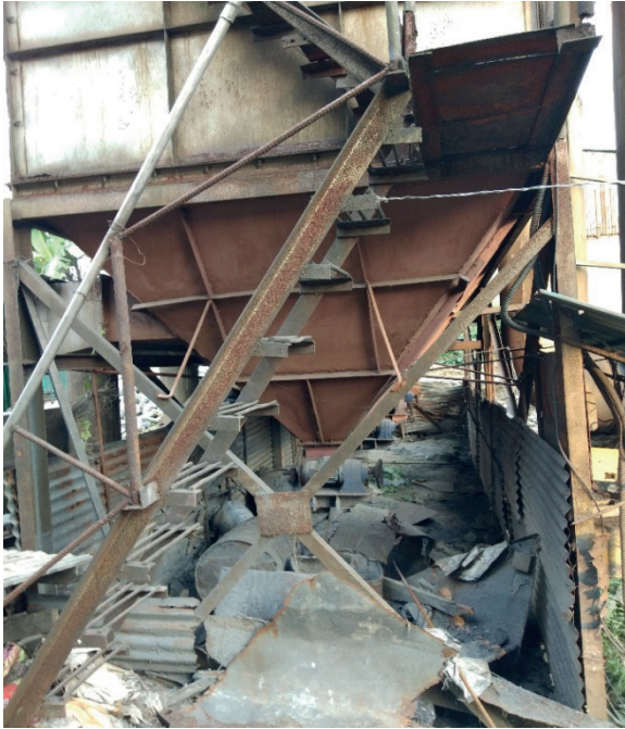
Figure 12: Junk lying below the Bag-filter hoppers at Lhaki Steel
