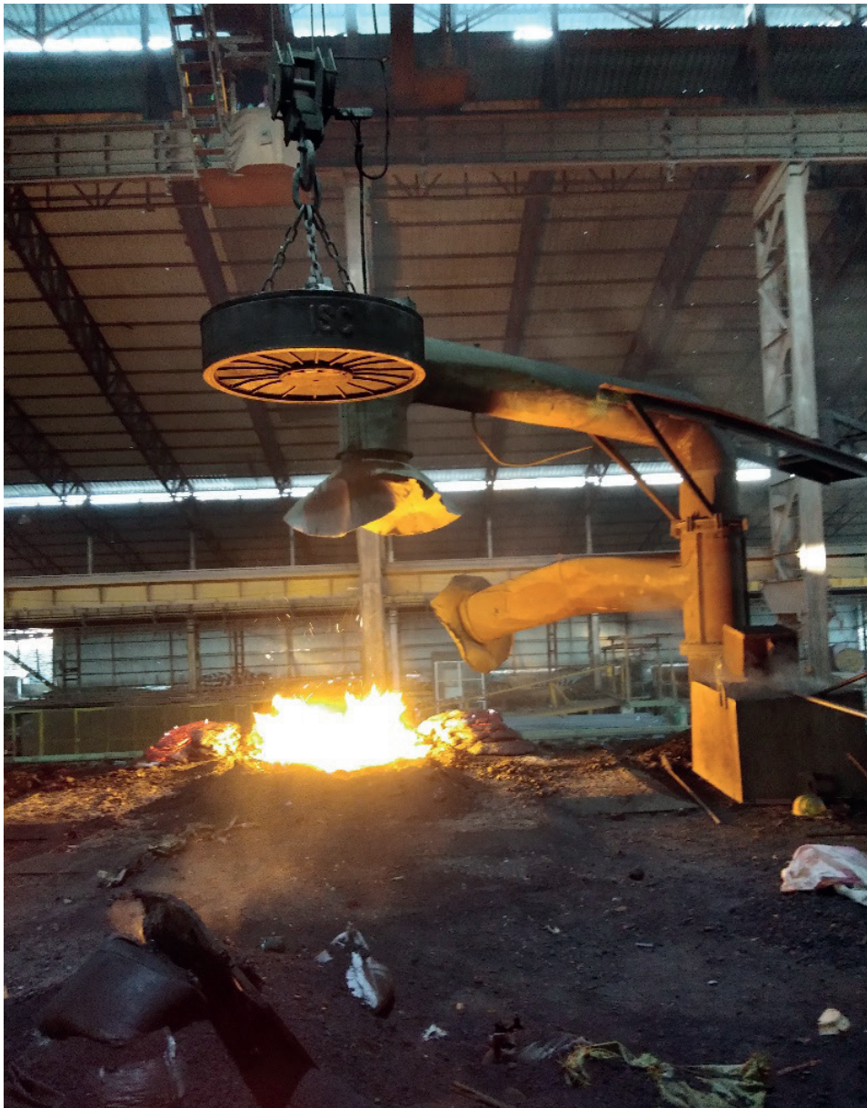
Figure 10: Inadequate Fume extraction system at Lhaki Steel and Rolling Mills
