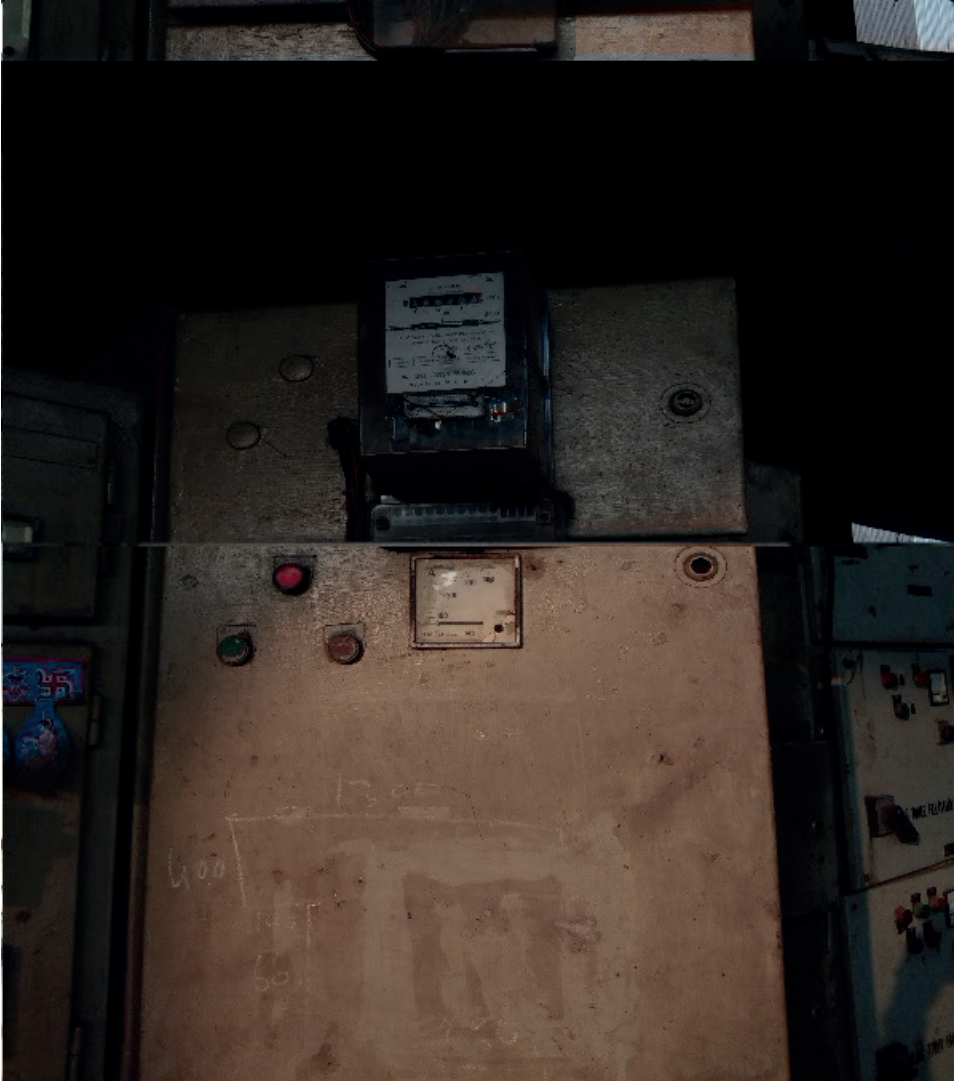
Figure 13: Analog energy meter at the fan motor of Lhaki Steel
