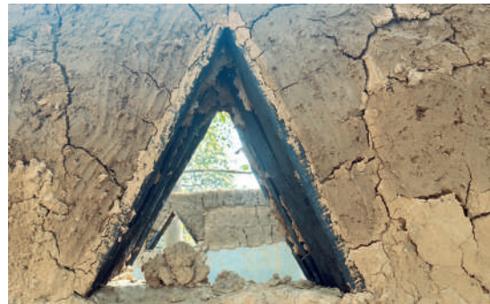
A wooden frame for triangular windows eliminates the requirement for a lintel
