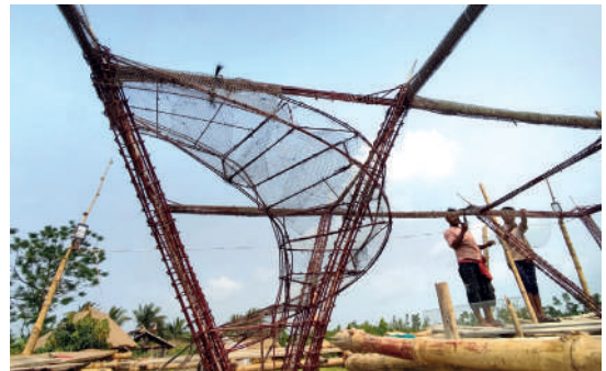
Stage 2: A layer of chicken mesh is used to make the reinforcement for staircases.
