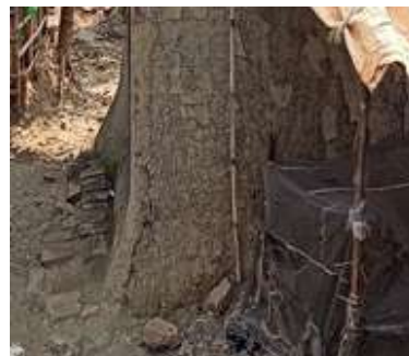
Impact of flooding on wattle and daub walls
