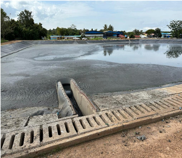
Anaerobic pond outlet to facultative ponds
