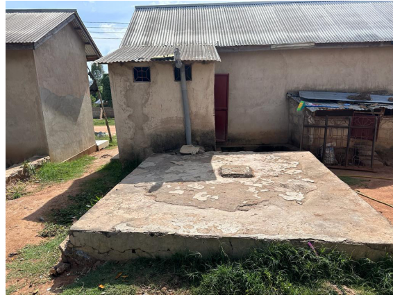
Sealed fully lined tanks in the Busewelu area
