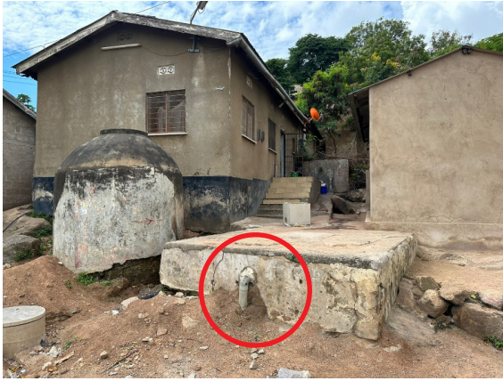
Fully lined tanks connected to the ground in the Ibungilo area
