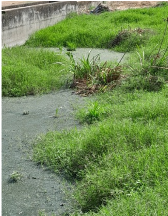
Unused anaerobic ponds with uncleaned sludge
