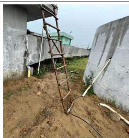
Photograph 13: Connection near sewage sump well
