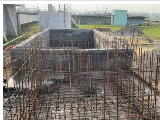
Photograph 10: Wrong construction of screen chambers
