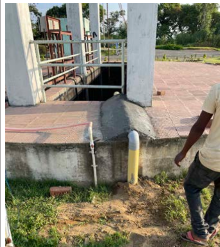
Photograph 15: Connection at inlet of STP
