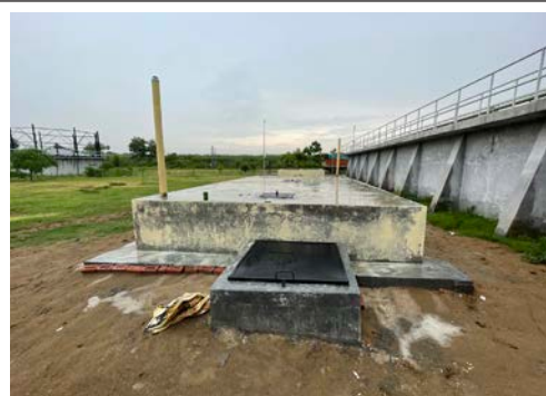
Photograph 8: Gas vent provided by the contractor
