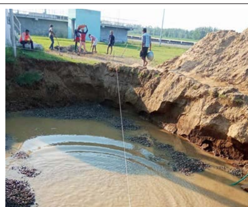
Photograph 7: Underground water coming to the surface
