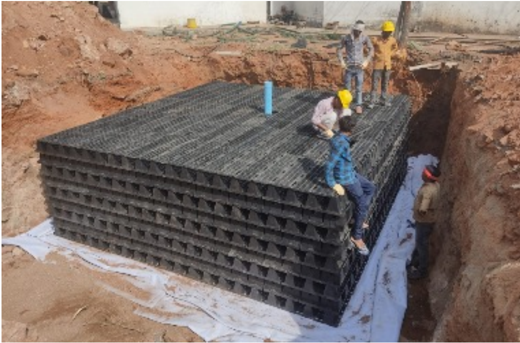
Photograph 29: Rainwater harvesting in Jhansi
