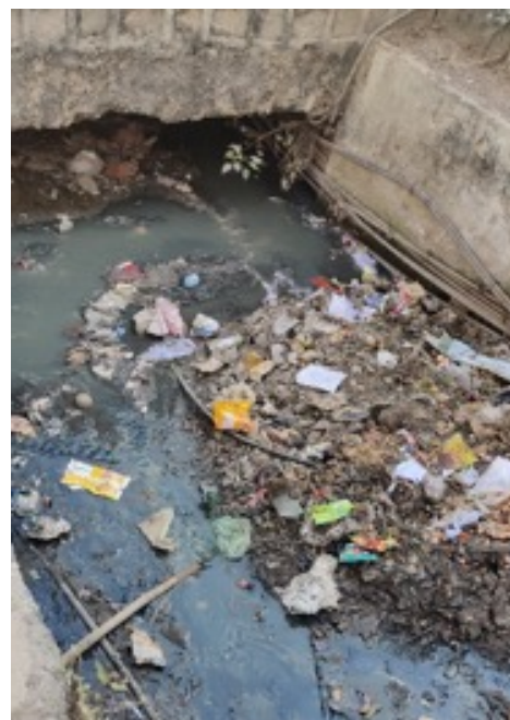
Photograph 33: Dumping of solid waste into open drains
