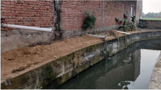
Photograph 20: Direct discharge of toilet waste into an open drain
