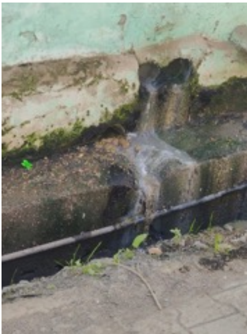
Photograph 32: Direct discharge of wastewater into an open drain in Bada Gaon area
