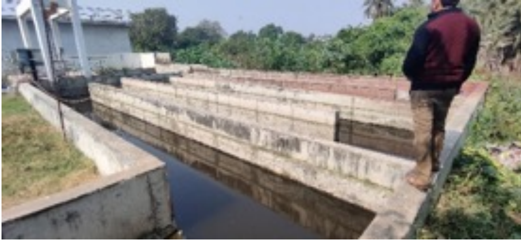
Photograph 17: Interception and diversion based STP of 26 MLD capacity
