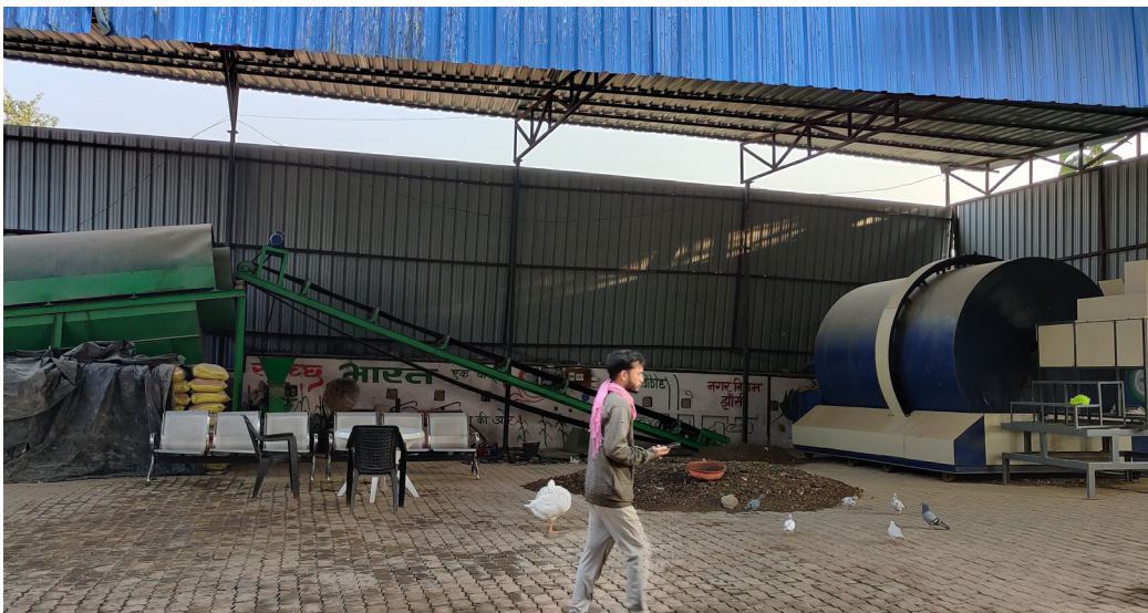
Photograph 6: Co-composting unit at Jhansi FSTP
