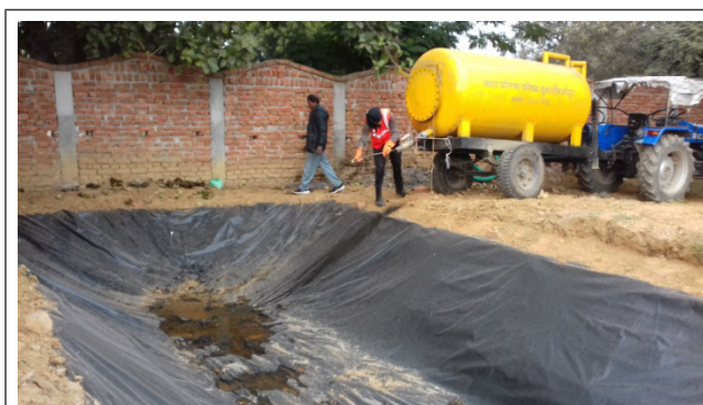
Photograph 7: Trenching in Chunar as an interim solution for safe disposal of faecal sludge
