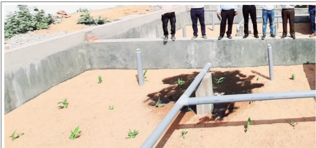
Photograph 14: Soft commissioning of the FSSTP
