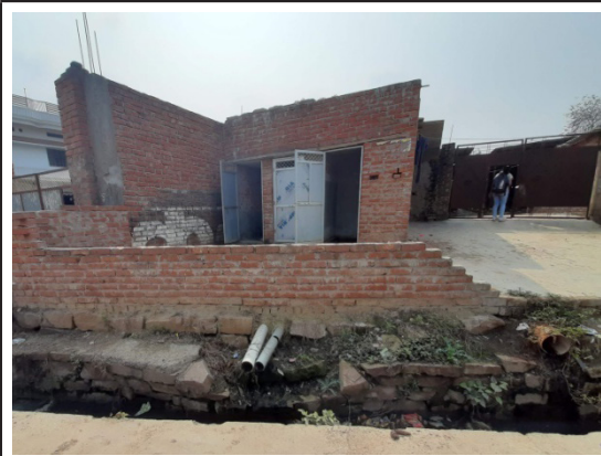
Photograph 2: Effluent from a septic tank flows into an open drain
