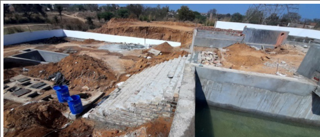
Photograph 12: Liquid treatment module
