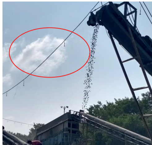
11b. Sprinkler not working near aggregate
