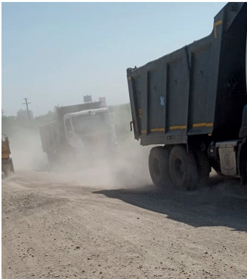
15c. Dust emission due to heavy vehicles
