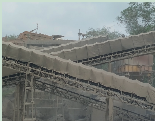
17b. Covered Conveyor belts
