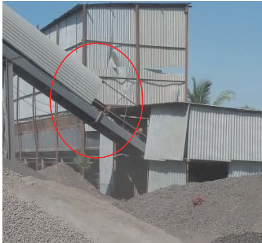
10a. Partially covered conveyor belts
