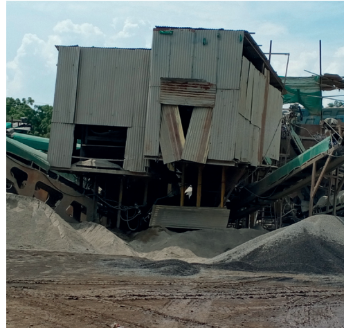
13b. Screen with inadequate covering
