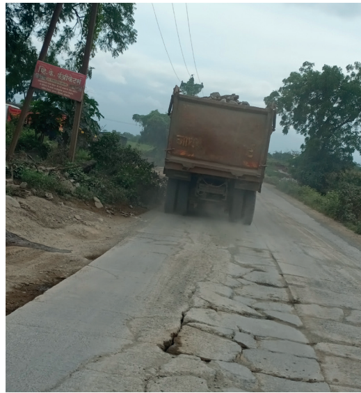
15d. Broken roads due to heavy vehicles
