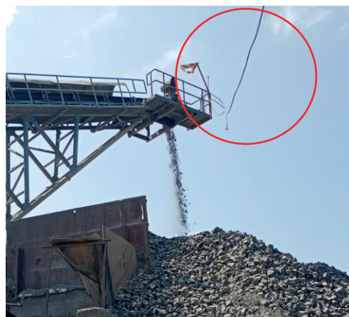
11d. Water sprinkler not working at heaps
