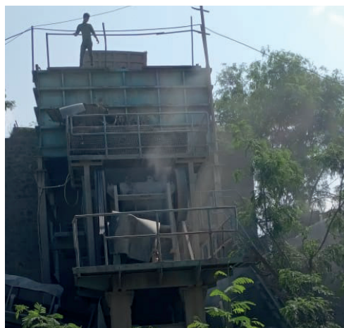
12b. Water sprinkler not working at hoppers
