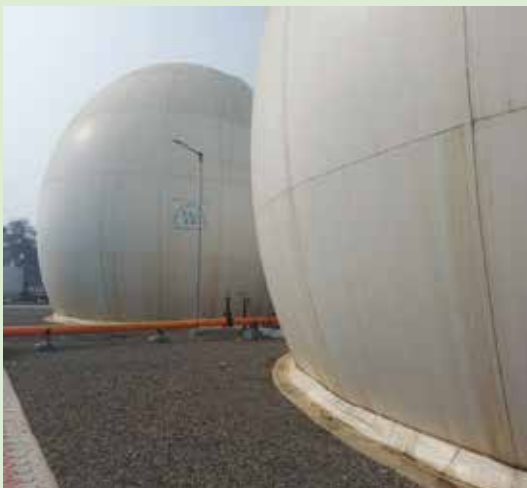
Biogas pipeline near digesters ▲
