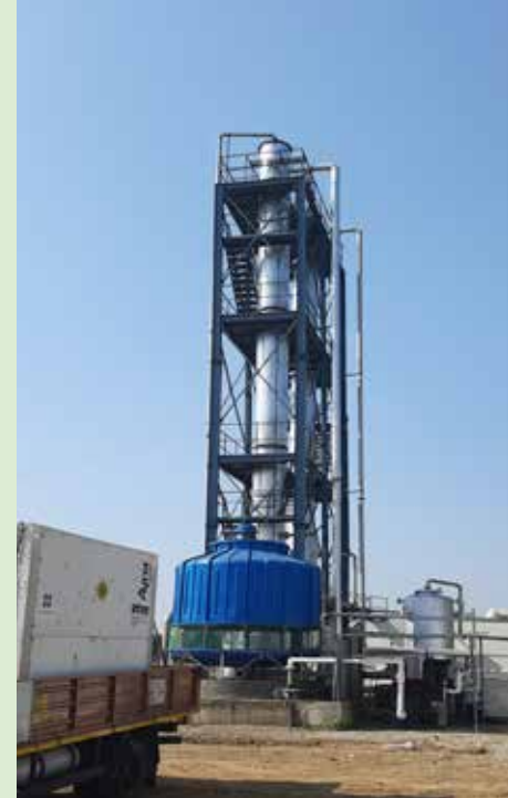
Water scrubbing unit ▲
