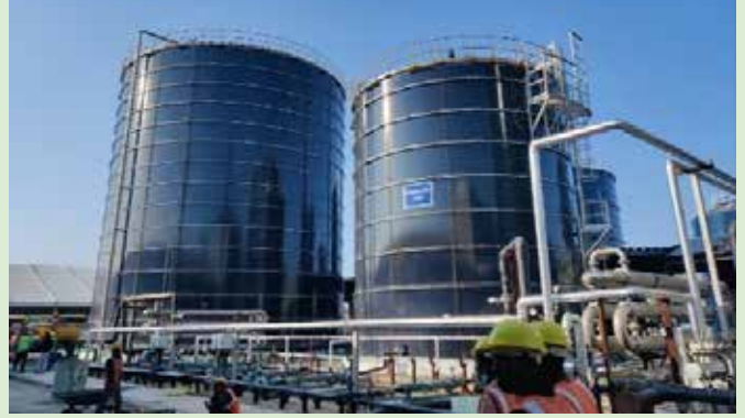
Anaerobic digestion units ▲
