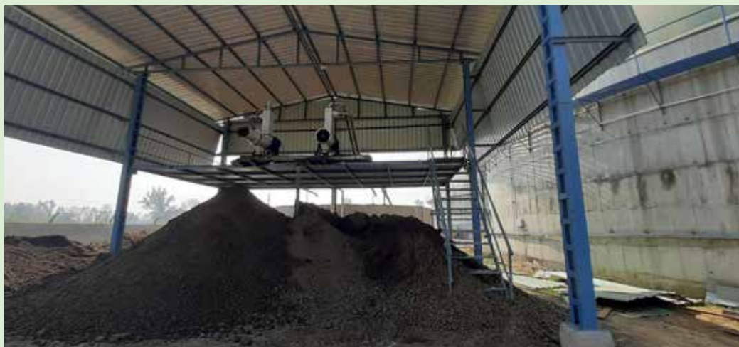
Biogas digester solid-liquid separator ▲
