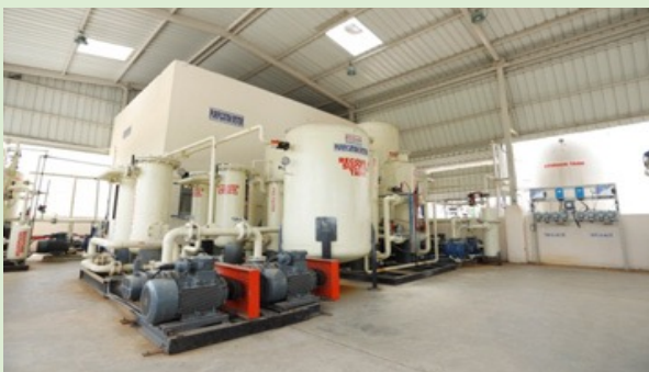
Biogas purification system ▲
