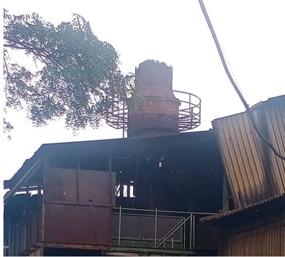
10b. Broken stack at a chimney
