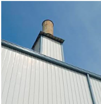
13a. Bag filter installed at the unit
