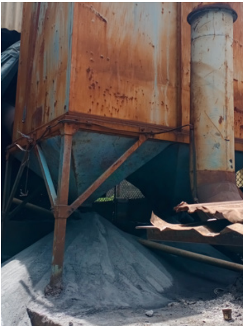
11c. Dust extraction system installed at unit
