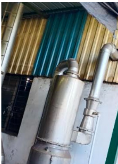
9a. Fume extraction system at a foundry
