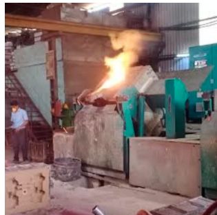
11e. Induction furnace installed at the unit
