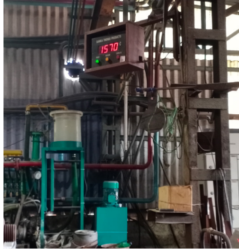
11b. Sensors to monitor temperature of molten metal
