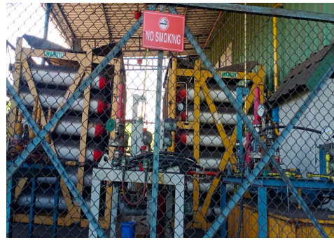
15d. Two sets of cascades for biogas storage
