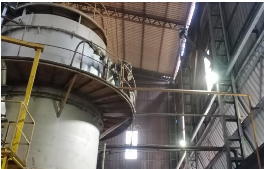
15c. Pipeline for PNG at thermal furnace
