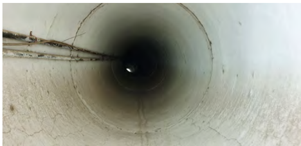
View inside the earth air tunnel
