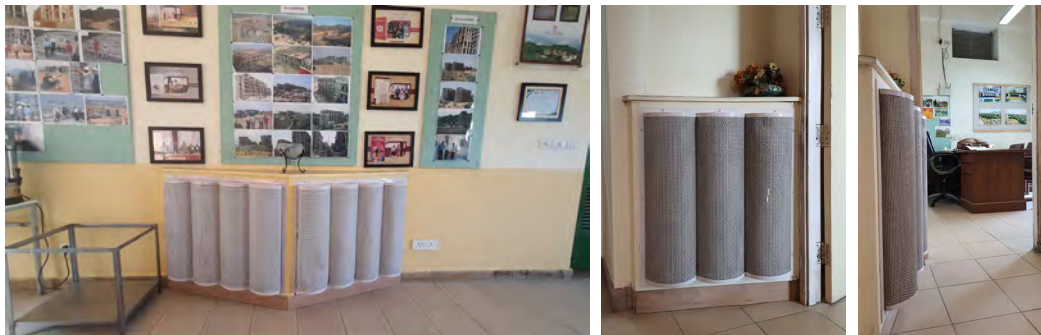
Inlets for conditioned air inside the building spaces.
