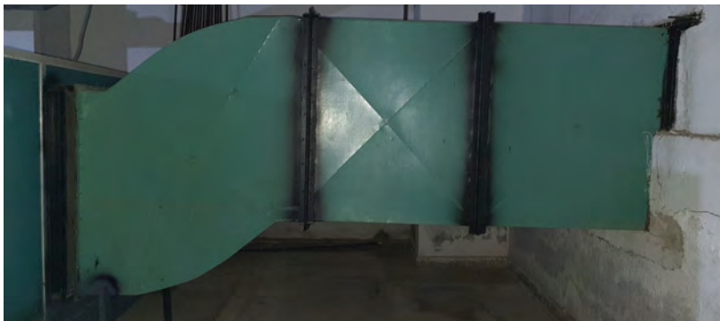
Duct joining the exit of earth air tunnel with other cooling stages
