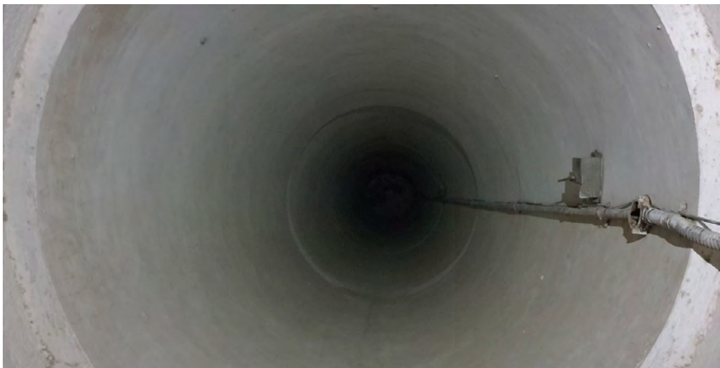
Earth air tunnel at NIIT University at Neemrana.
