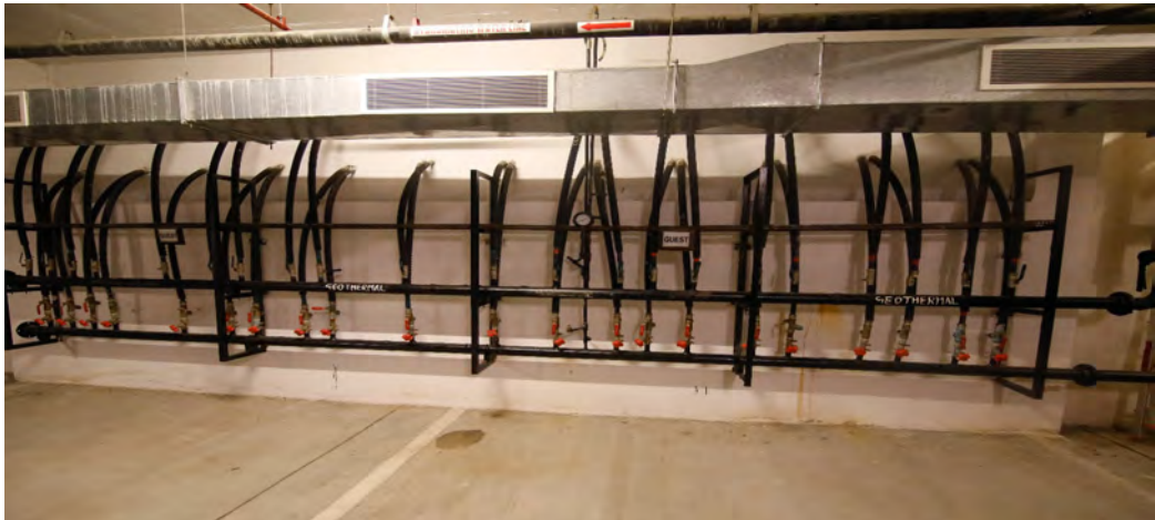
Geothermal wells installed in Norwegian embassy helping in heat rejection by HVAC system.
