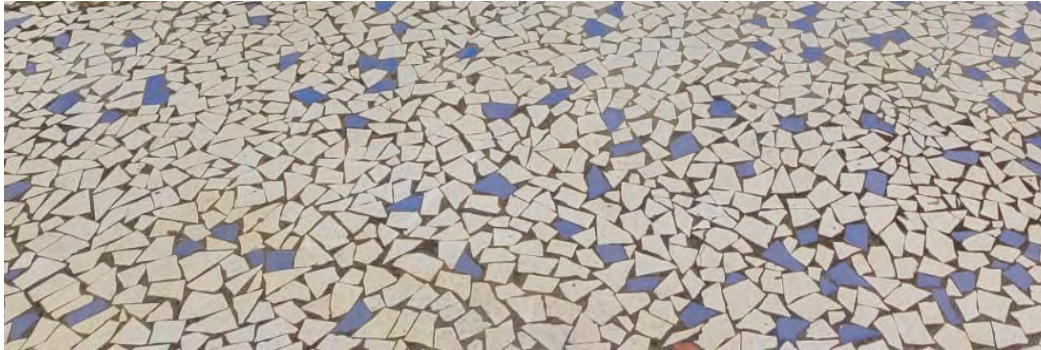
White shiny ceramic tiles of 13mm thickness cover the roof of buildings as they reflect the harsh sun rays and reduce heat gain. The roof also has a 100mm of XPS insulation below the ceramic tiles.
