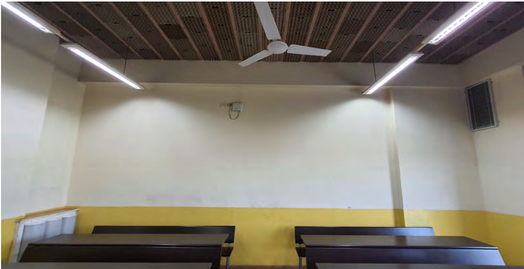
Interior of classroom with an inlet in the bottom left and outlet at the top right
