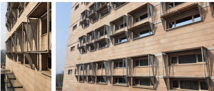
The glass used for the windows is high-performance double-glazed-units with vacuum to offer good insulation.
