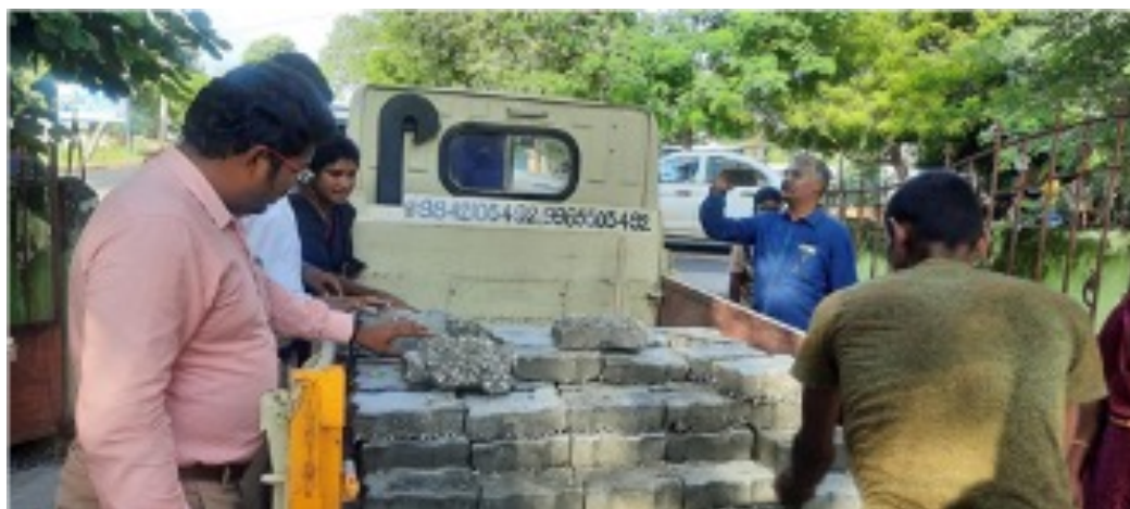
Photograph 23: Some plastics are visible in the paver blocks
