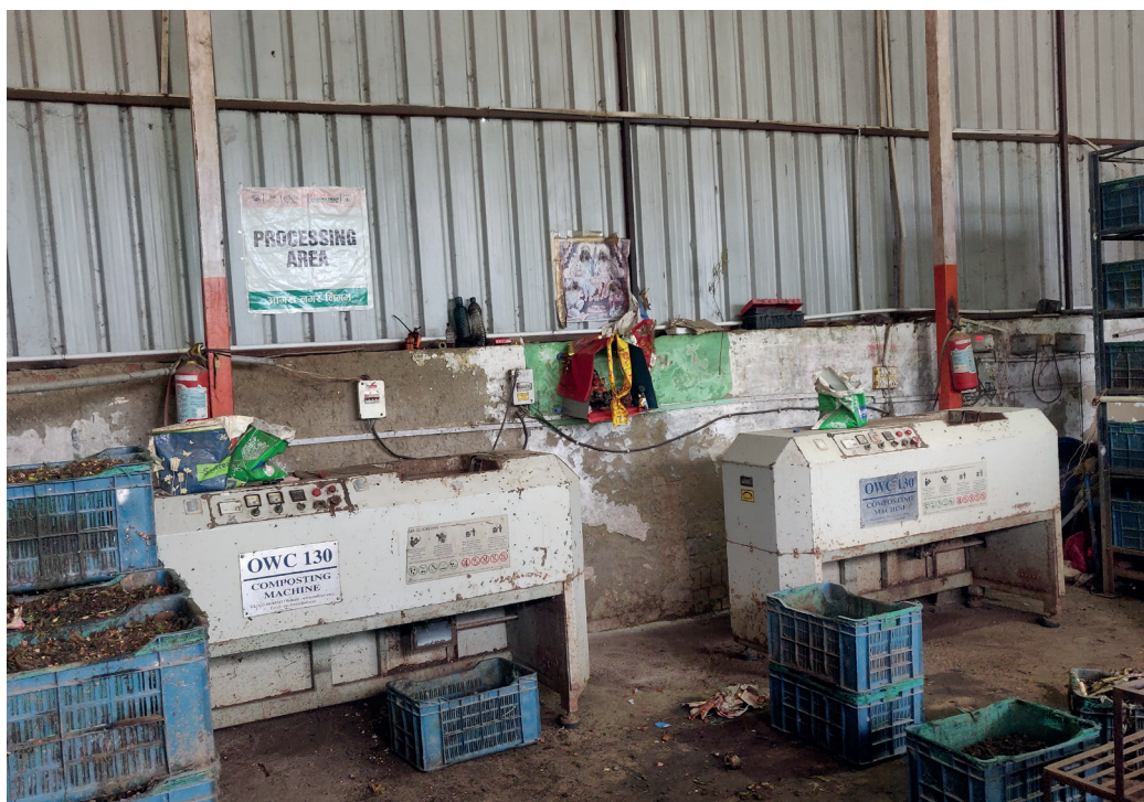
Photograph 13: Raj Nagar organic waste to compost plant
