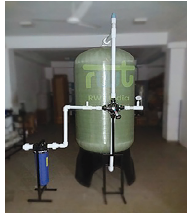
Figure 9: Pressure sand filter (PSF)
