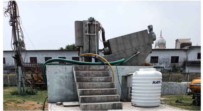
Co-treatment facility in Ayodhya
