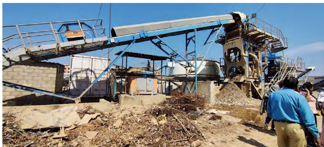
Cone crusher unit further breaks down the particles and takes them to a dewatering screen, where coarse and fine particles are separated
