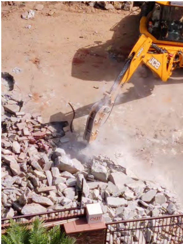
Demolition activity near India Habitat Centre resulting in debris and fugitive dust
