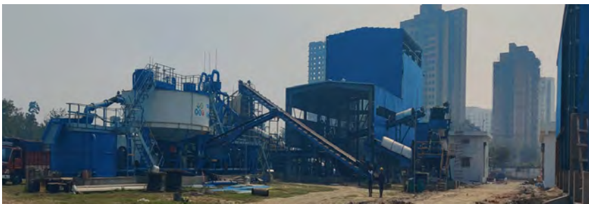
C&D waste processing plant
