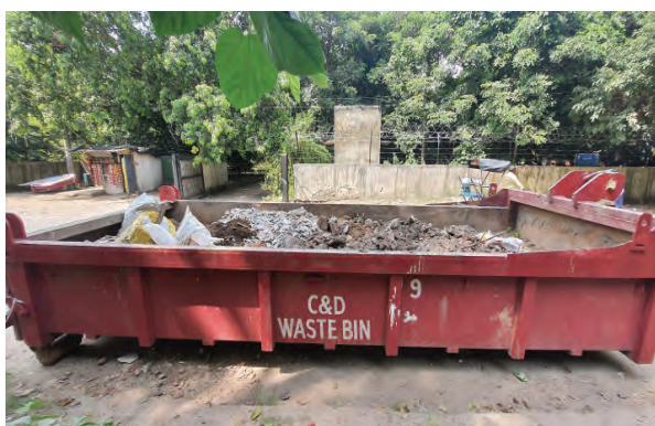
C&D waste collection point under New Delhi Municipal Council
