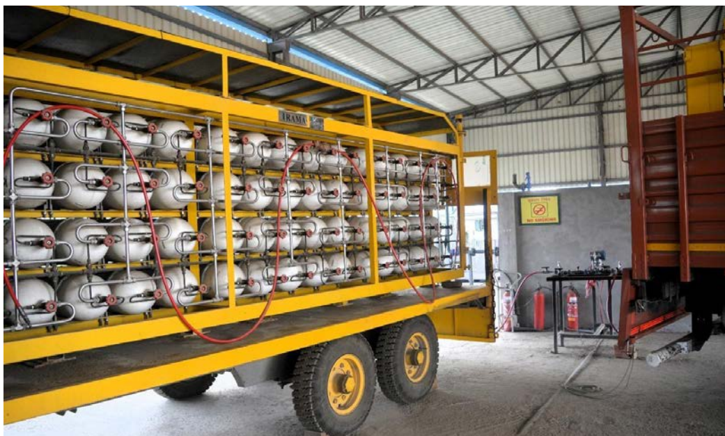
Image 6: Offtake of CBG gas from the production plant using cascades
