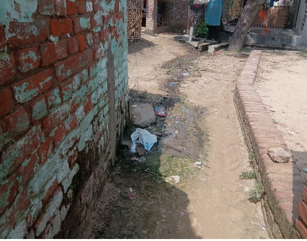
Lack of drainage results in waterlogging outside houses where households manage with temporary arrangements in Jahanpur Kodar village, Rahi block.
