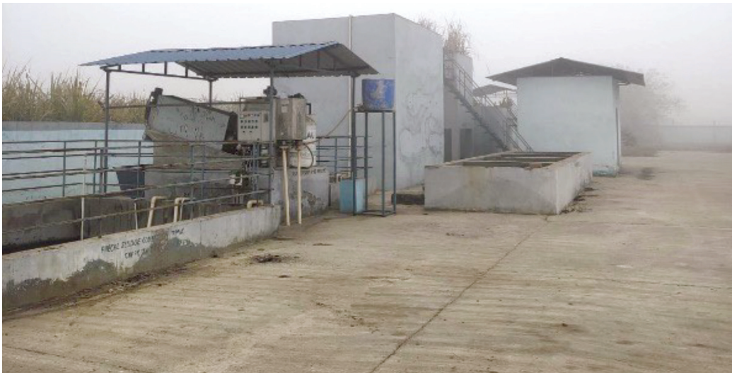
Primary stage treatment facility in Shamli
