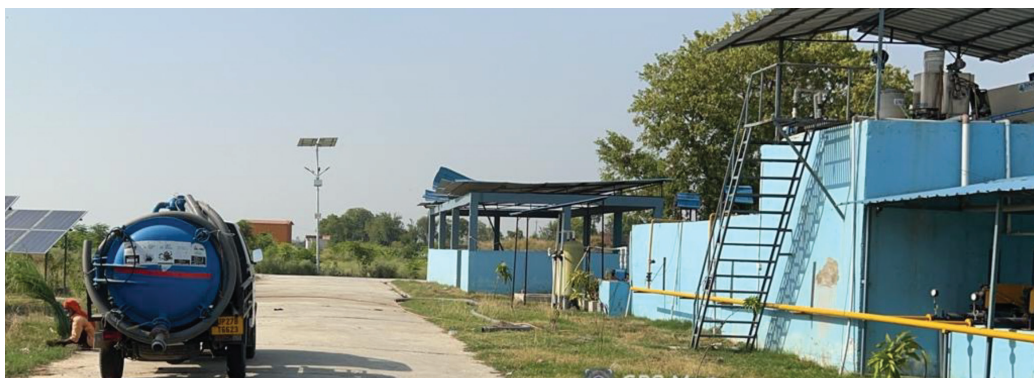
Primary and secondary stage treatment in Shahjahanpur
