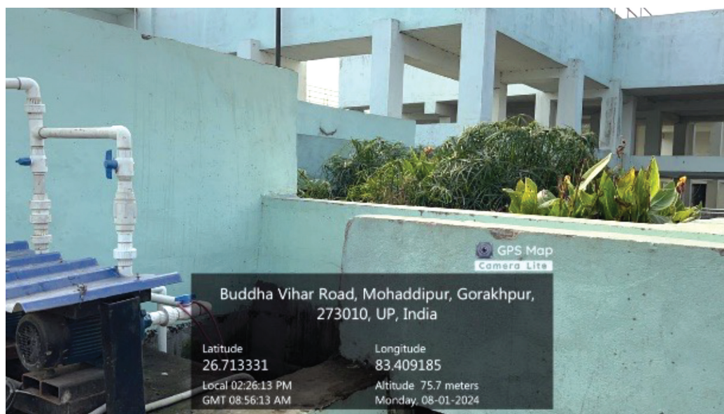
The Gorakhpur plant's primary treatment facility
