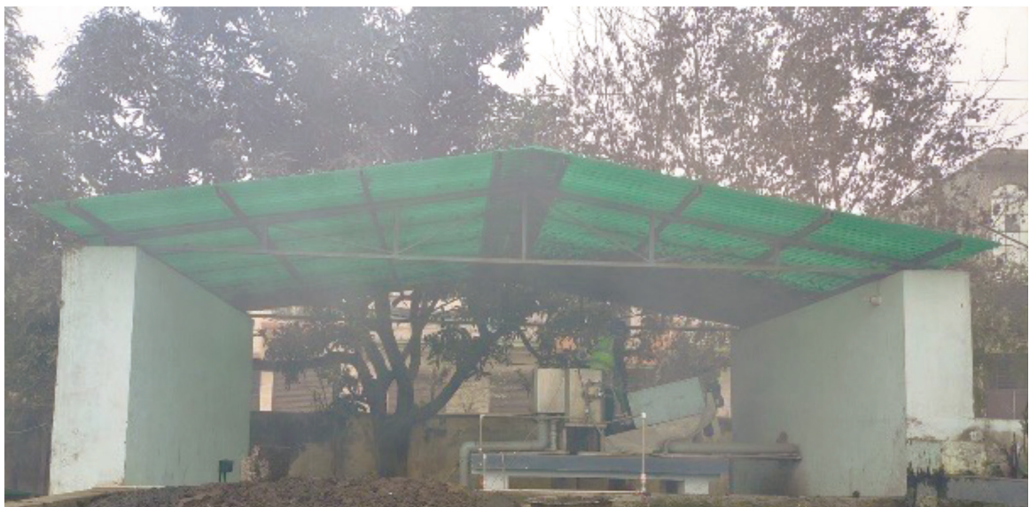
The primary treatment stage and drying bed in Saharanpur
