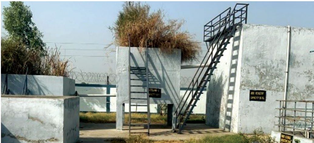
Primary and secondary stage treatment in Hapur
