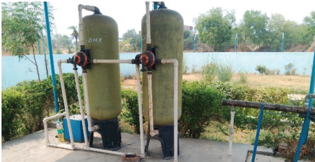
Filtration module in the Chunar plant
