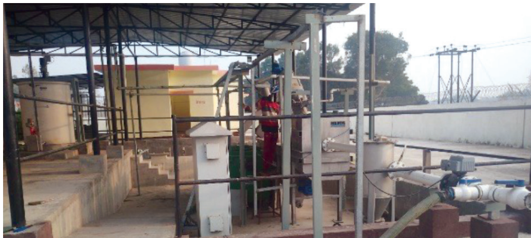
Preliminary stage of the treatment module in Basti
