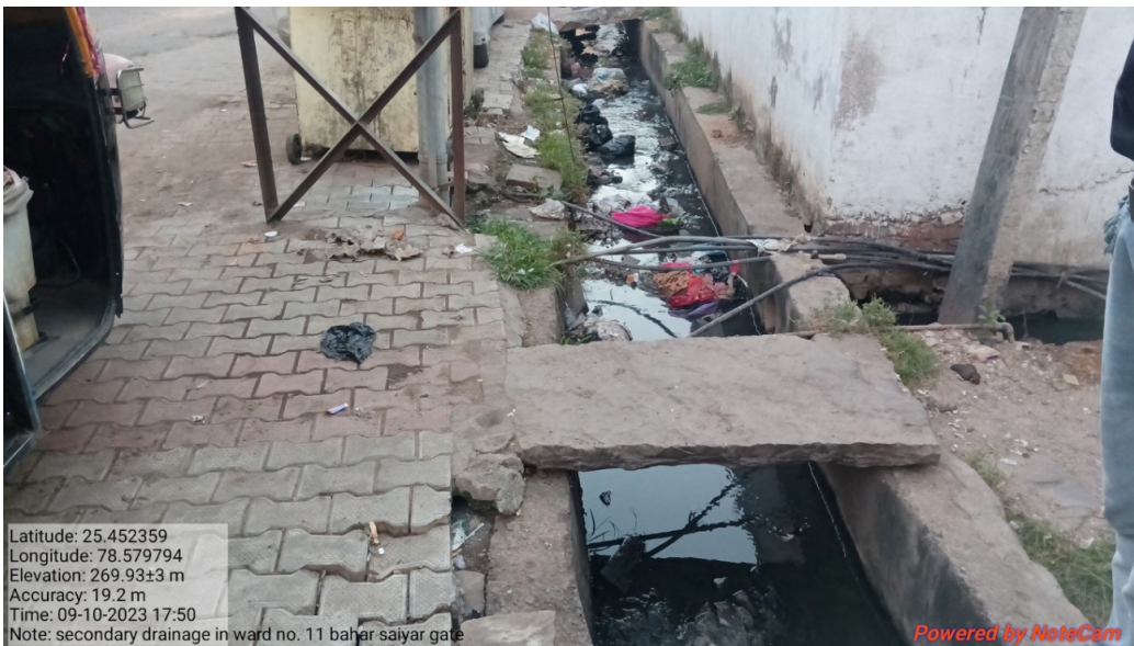
There is no management of the solid waste in the city. Solid waste is dumped everywhere, including in storm-water drains. The drain in ward number 11 is a good example of drains choked with solid waste, especially plastics.
