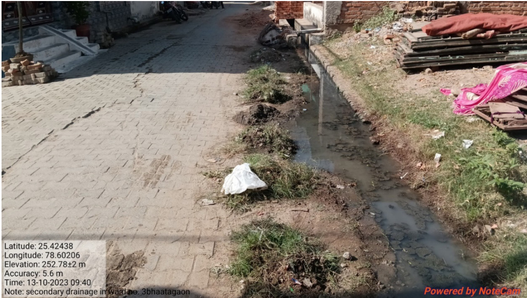
The storm-water drains in most of the wards of Jhansi are poorly built and broken, and spill over even after light showers
