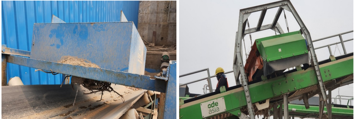
Image 28: Overhang magnetic separator installed at Greater Noida (Left) and Over band magnetic separator in Burari, Delhi (Right)
