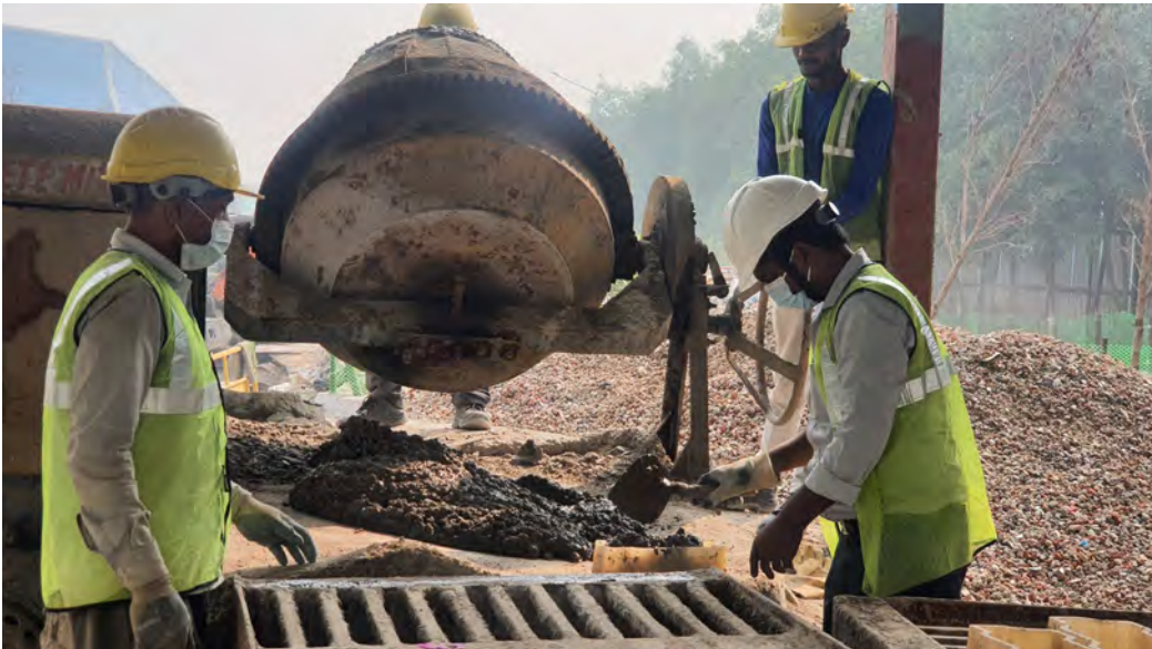
Image 38: Concrete mixture unit
