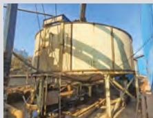
Thickening tank/Water recycling tank Approx. cost: Rs 1-2 crores
