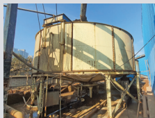
Thickening tank/Water recycling tank
