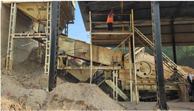
Image 22: Grizzly screen at Chandigarh C&D recycling plant
