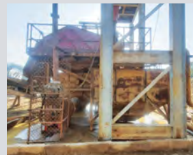
Hydrocyclone Approx. cost: Rs 1-1.5 crores
