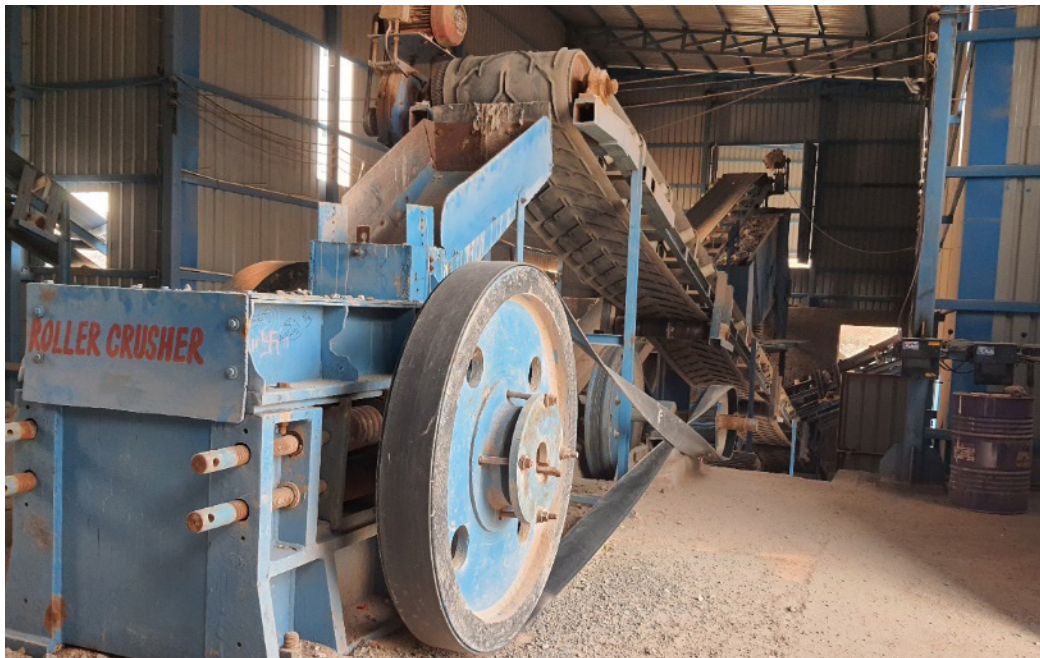
Image 24: Roller crusher installed at Greater Noida C&D recycling plant
