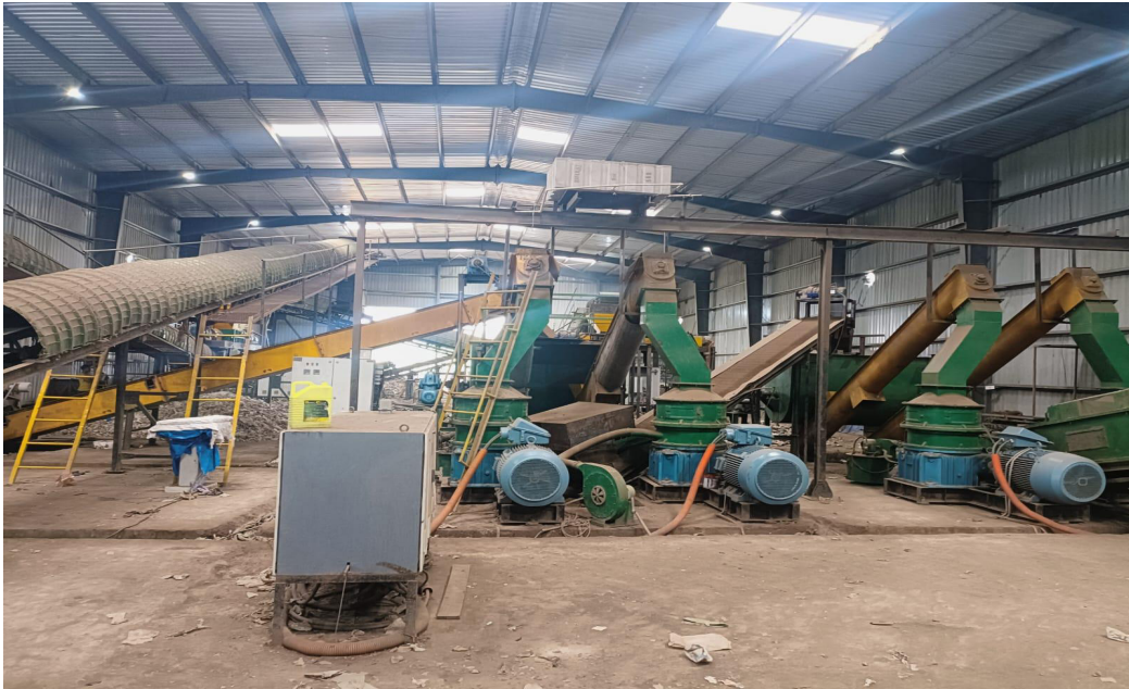
RDF pelletization plant at Mulund dumpsite in Mumbai
