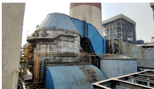
Absorber tank of FGD at Jhajjar Power
