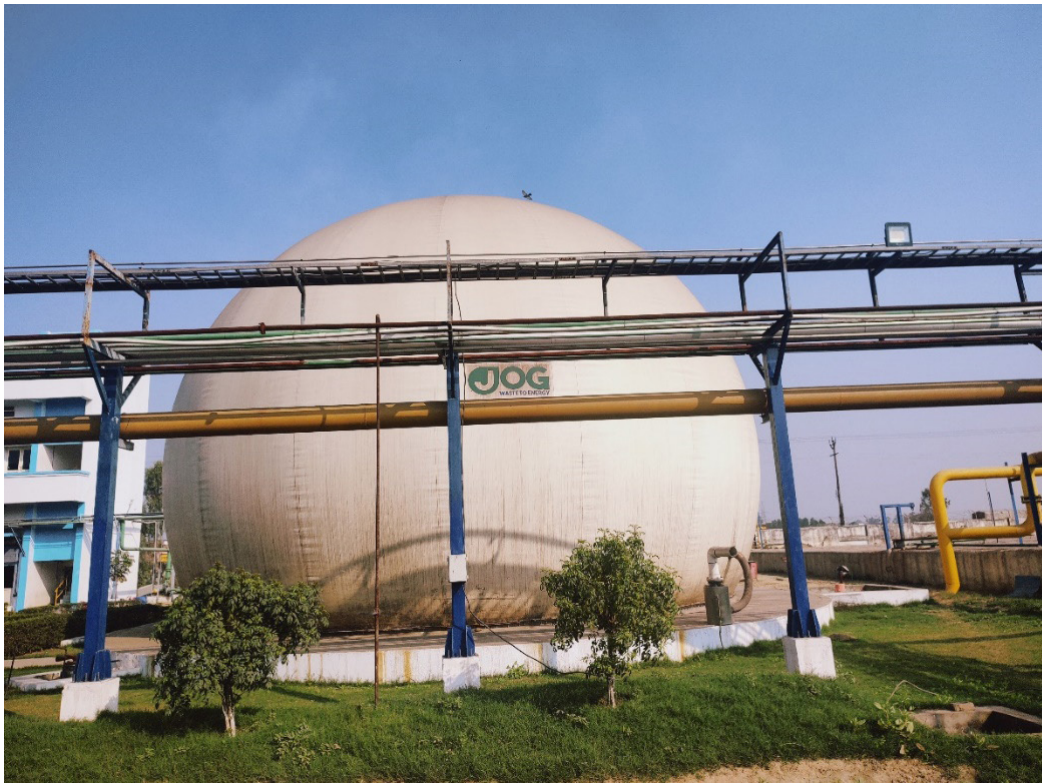
Compressed biogas plant in IPL
