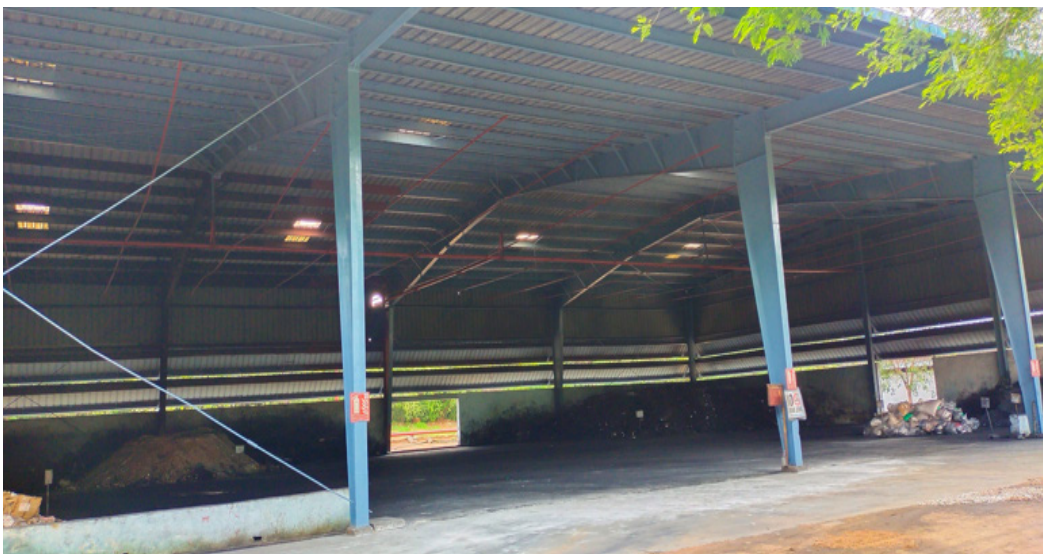
Storage of processed alternative fuels and raw materials (AFR) under a shed
