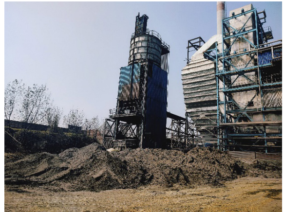
Fly ash from boiler of sugar mill
