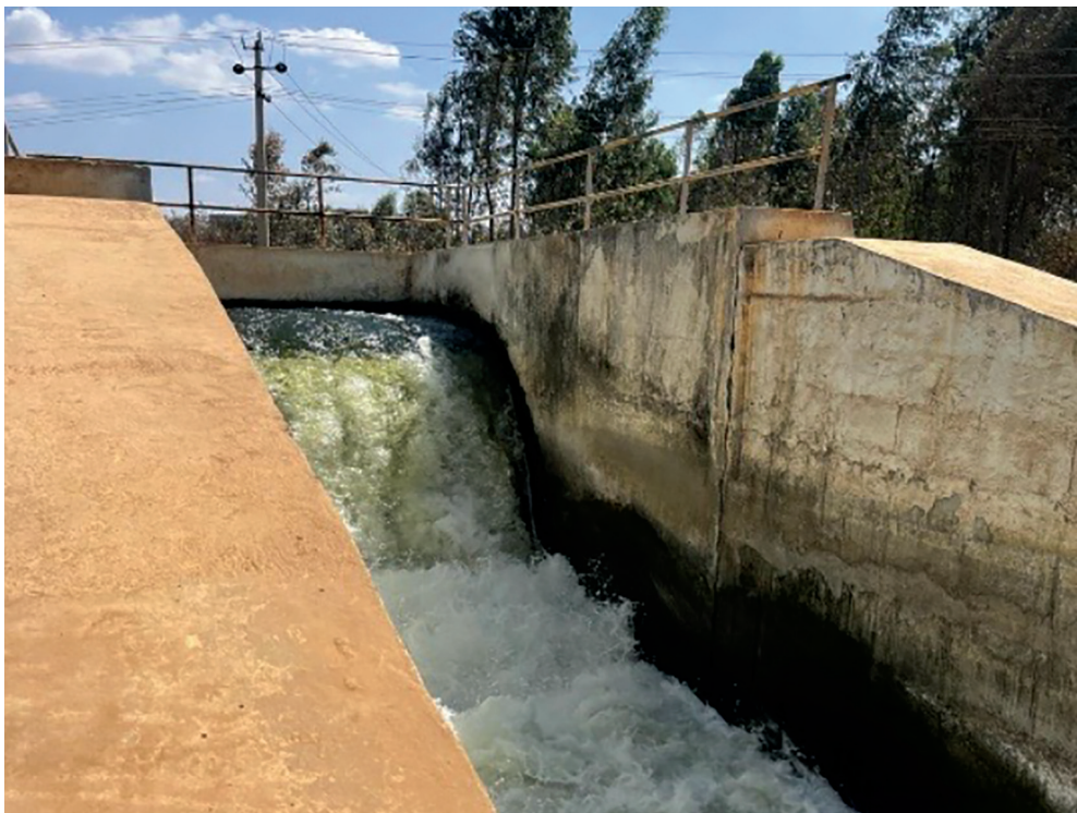
Inlet point from where the treated water from Hebbal, Rajacanal and Horamavu STP is getting released in Bagaluru Lake.
