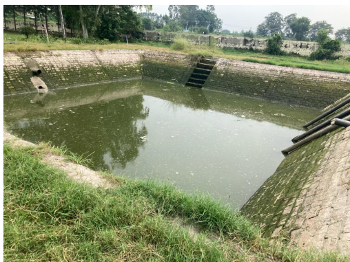
Constructed reservoir to store the treated water in the premises of Ladwa STP
