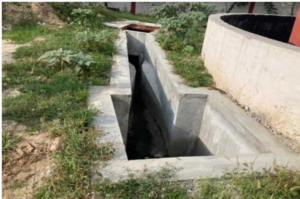
Escape channel in 1.5 MLD treatment plant in Beawar for disposing treated water to the pond adjacent to boundary of the plant.
