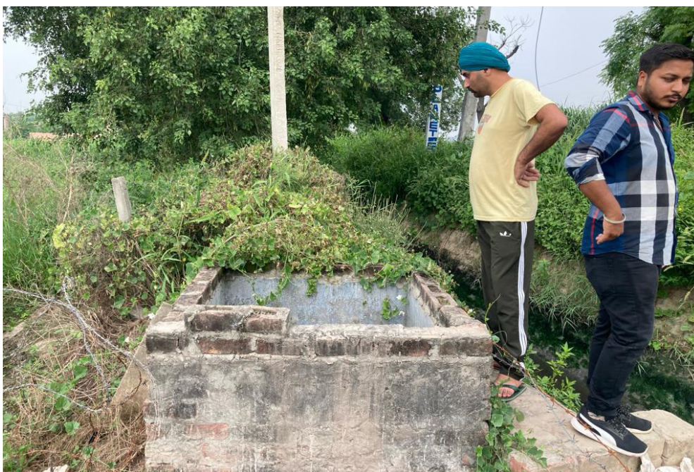
Chamber constructed by farmer where the treated water enters from the canal which is then used for agriculture in Chhapra village, Kurukshetra district, Haryana
