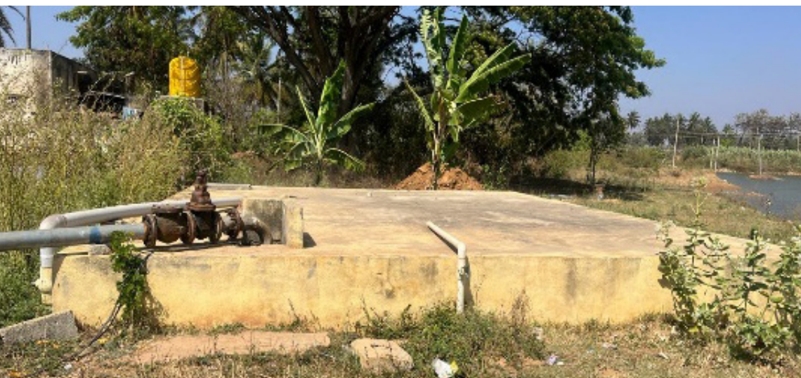
Sump to store the water after treatment
