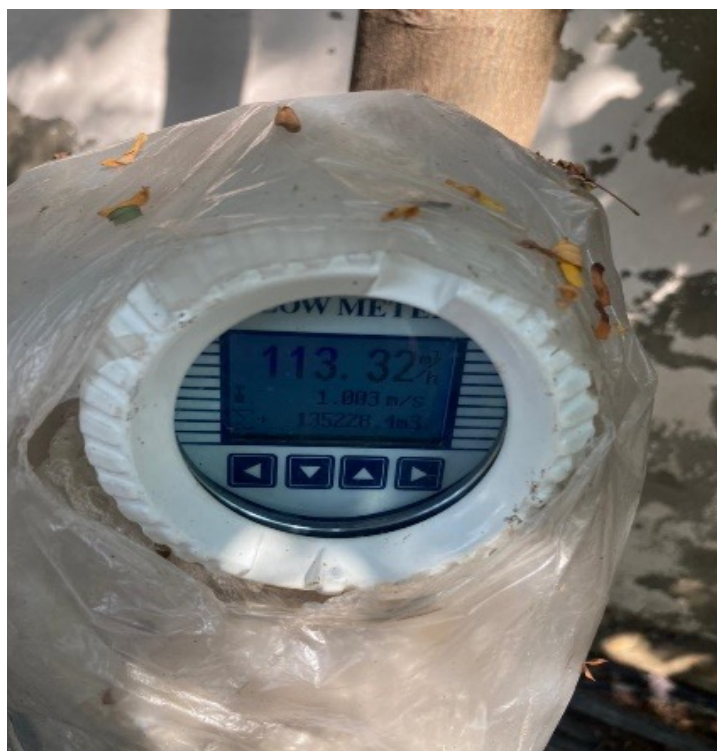
Flowmeter installed in plant to monitor the quantity of water pumped to SCL
