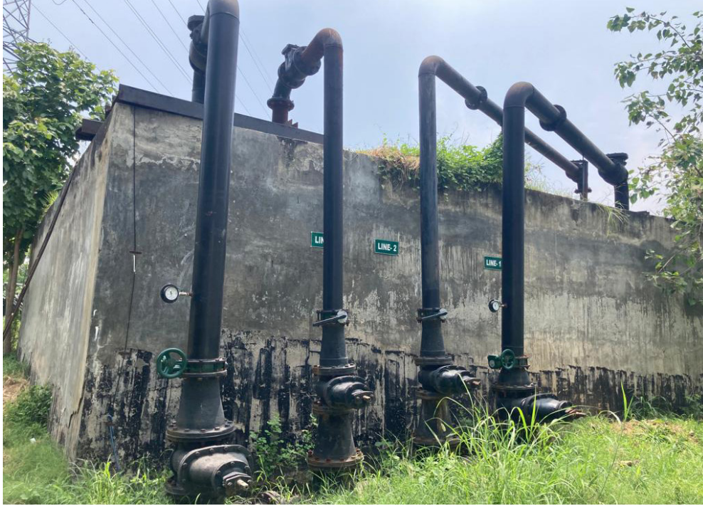
Existing pipeline network at Behrampur STP used for supplying treated used water for textile industries in Sector 34, Gurugram
