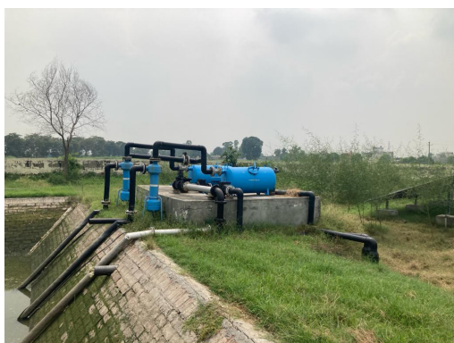
Pumping infrastructure with sand filters to distribute water for irrigation in Baraichpur village, Kurukshetra district, Haryana.
