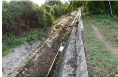
Naini channelo for distribution of treated wastewater for agriculture from Naini STP
