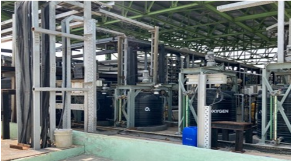
Tertiary treatment unit of 20 MLD at Lakshminagar in Mathura
