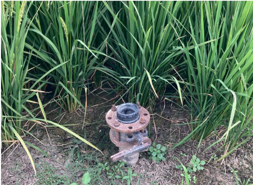
Hydrant installed in the field of farmers for treated water supply in Chhapra Village, Kurukshetra district, Haryana.
