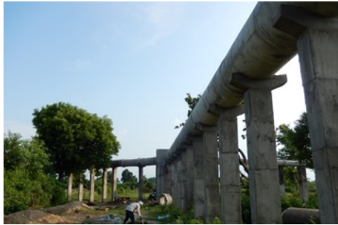
Dandi channelo for distribution of treated wastewater for agriculture from Naini STP
