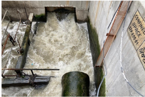
Inlet point for receiving sewage water at Eklingpura STP, Kaladwas village, Udaipur
