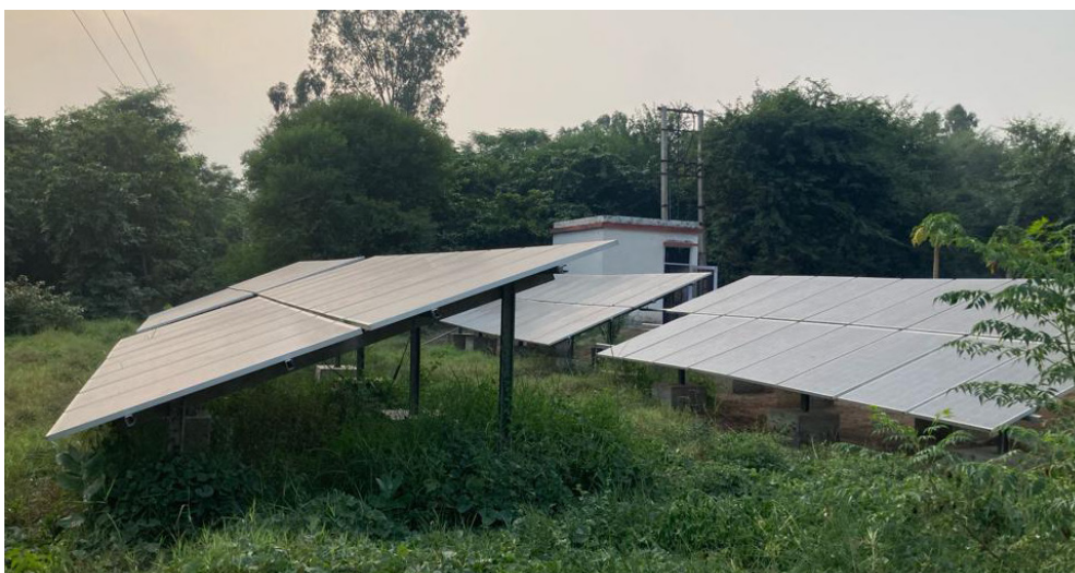
Solar panel installed in Pehowa STP premises to supply energy for pumping water for distribution in nearby villages.
