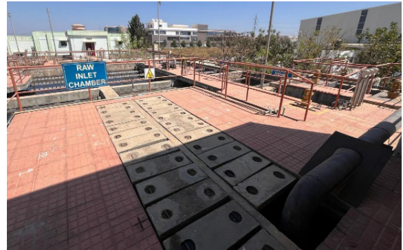
Raw inlet chamber to receive secondary treated water from Raja Canal STP at IT Park Industrial Area
