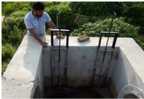
Access point on Dandi channel fro farmers to collect water
