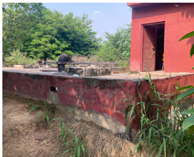
Underground tank of 0.5 MLD capacity for storing treated water for horticulture purpose in Tau Devilal Stadium, Sector 38, Gurugram
