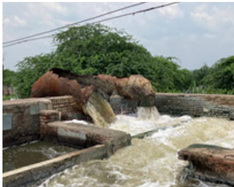
Treated effluent outlet of Jajmau, STP flowing in escape canal, Kanpur
