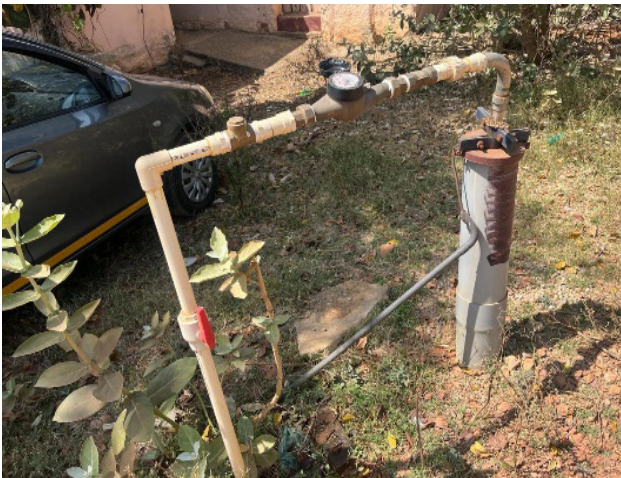
Filter borewell near Sihineeru lake for water supply
