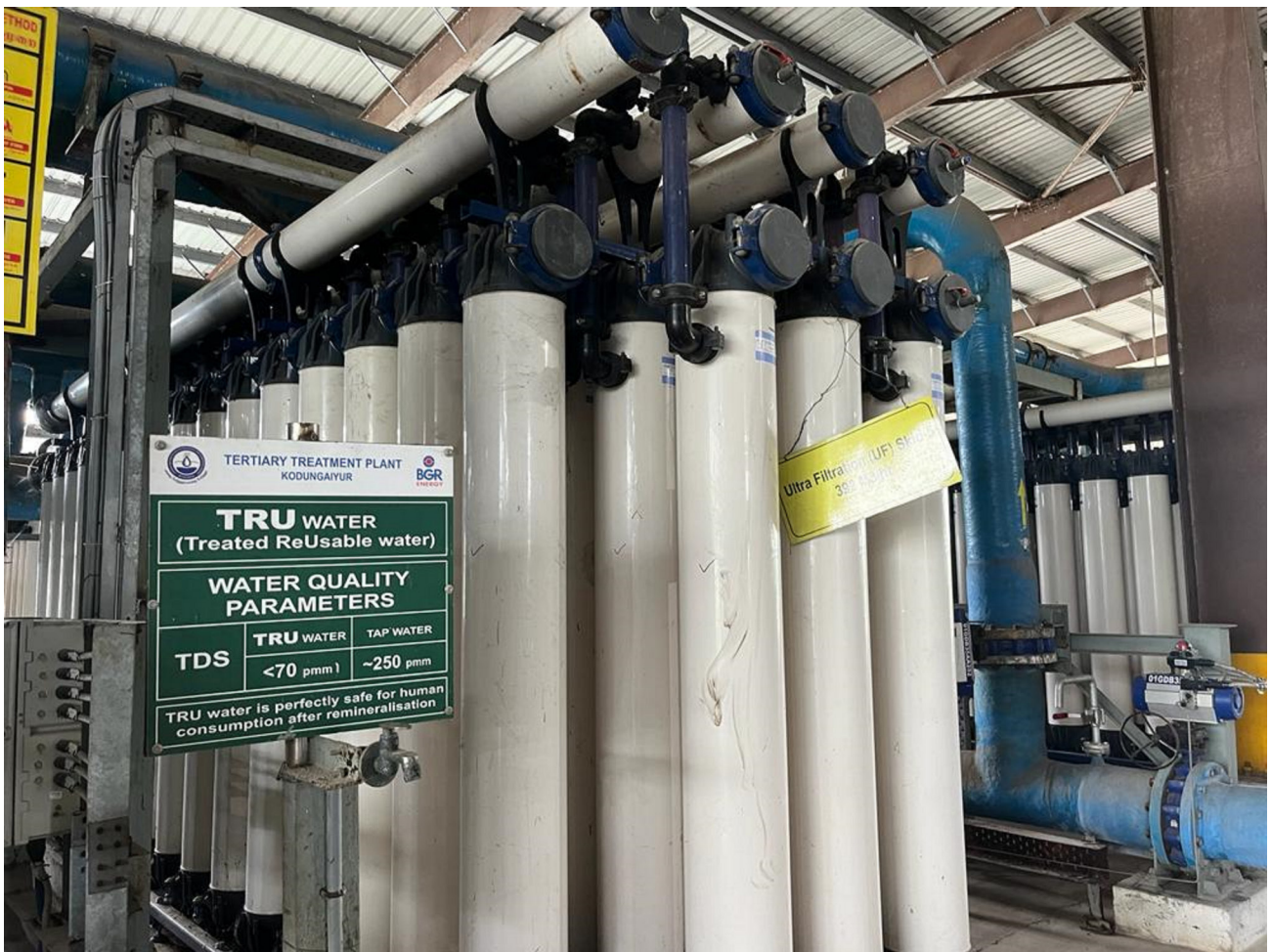
Tertiary treatment plant in Kodingaiyur, Chennai from where the treated wastewater is supplied for industrial reuse.
