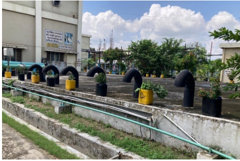
Tank constructed at Eklingpura STP, Kaladwas village, Udaipur where treated water is stored for further use.
