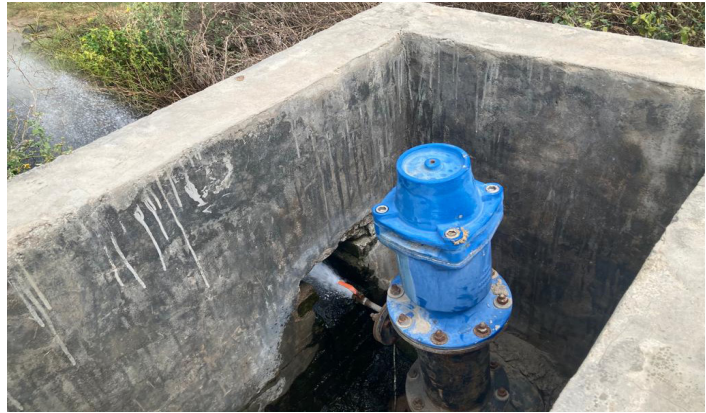
Hydrant at Sakatpur road (leopard trail) in Gurugram through which supplied treated water is discharged in water bodies for restoration.
