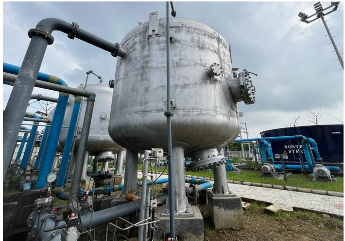
Water treatment plant of 6 MLD capacity which sources the inlet water from Porur lake. Water treated from this plant is supplied to Chennai city for non-potable use.
