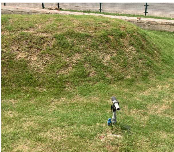
Smaller hydrant (access point) near Almeda Chowk, Sector 70, Gurugram from where the treated water is used for horticulture
