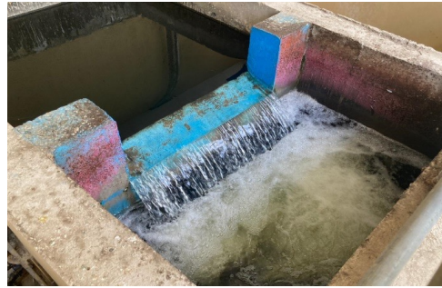
Outlet point of treated water at Eklingpura STP, Kaladwas village, Udaipur designed for its disposal, after which it is transferred to storage tanks for further use.
