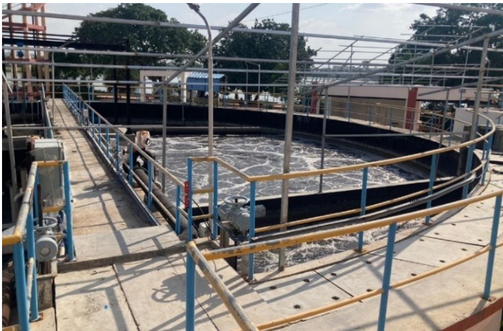
5 MLD Sewage Treatment Plant, Bewar, Rajasthan
