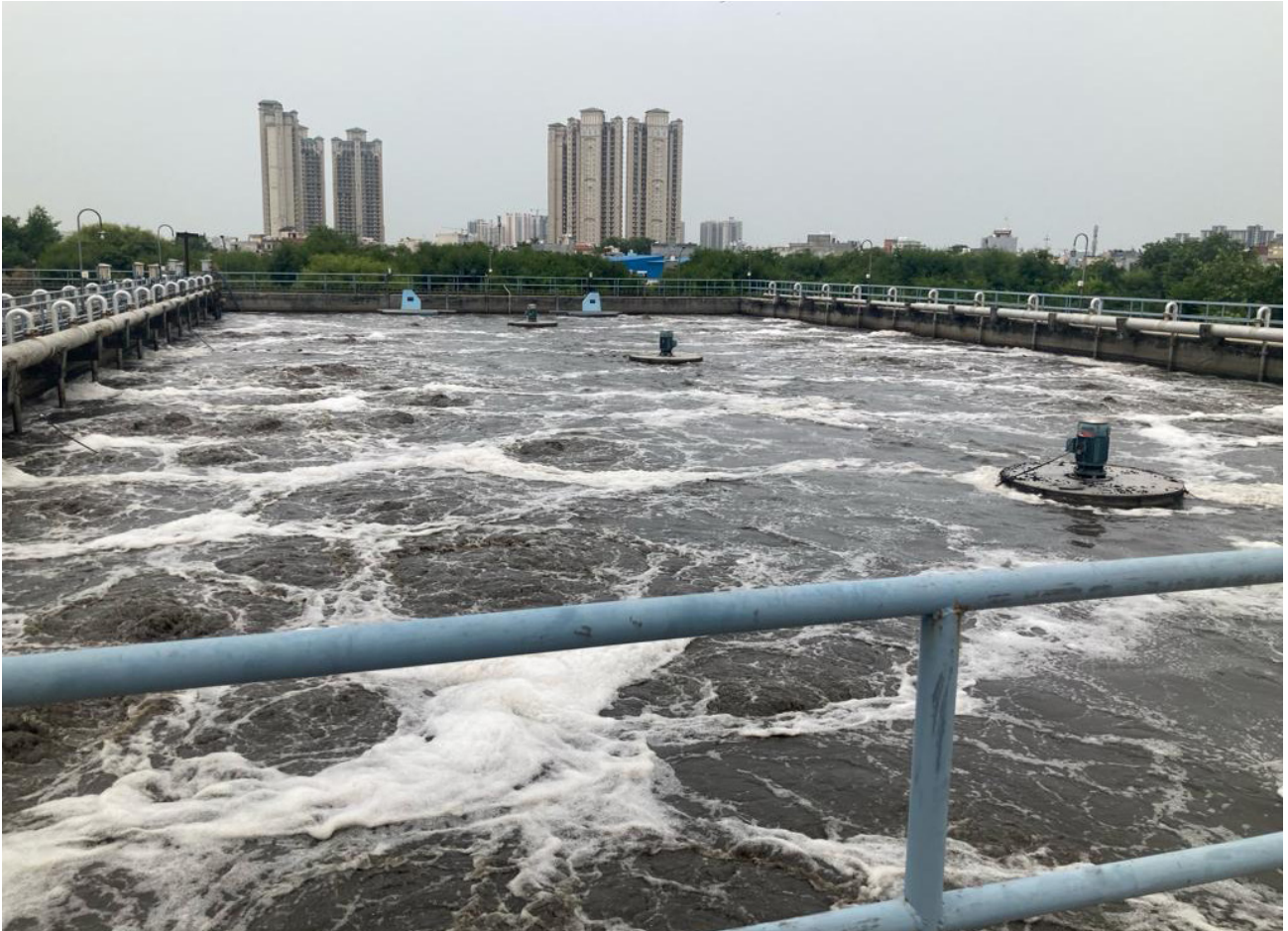
Dhanwapur Sewage Treatment Plant in Gurugram, Haryana. The total treatment capacity of this plant is 218 MLD.
