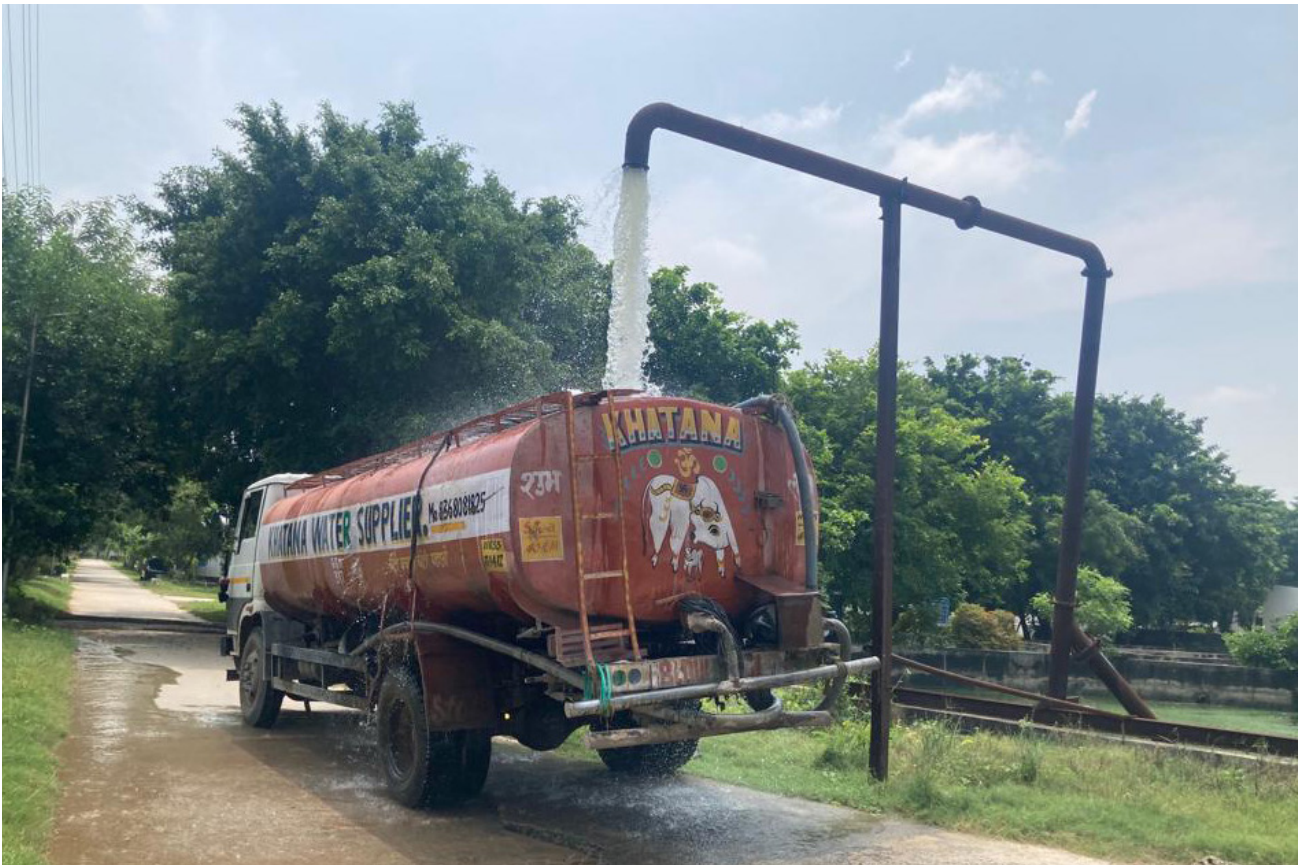
Tanker getting filled with treated wastewater for reuse in construction activities from hydrant located inside Behrampur STP
