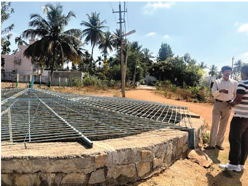
Revived open well near Sihineeru lake for shallow aquifer recharge and to supply water
