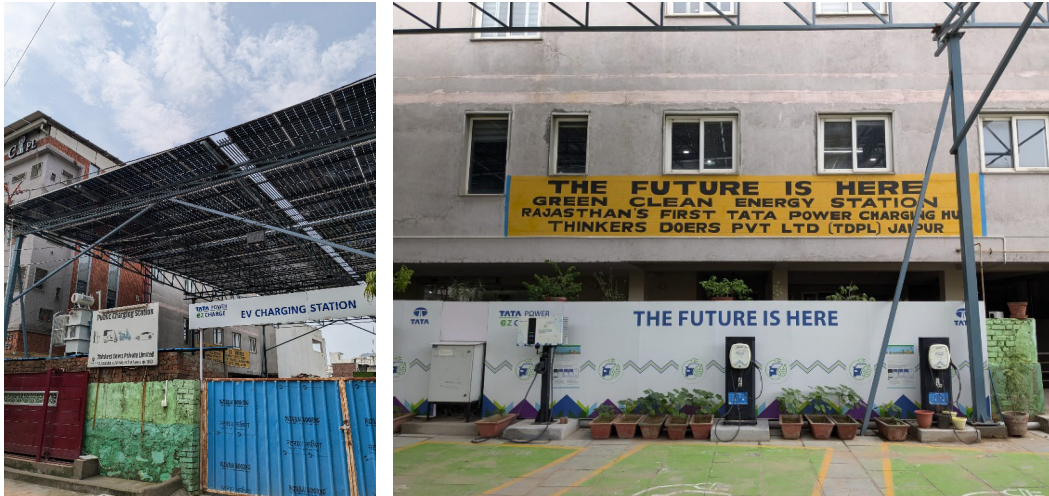
Figure 5: Solar powered EV charging station
