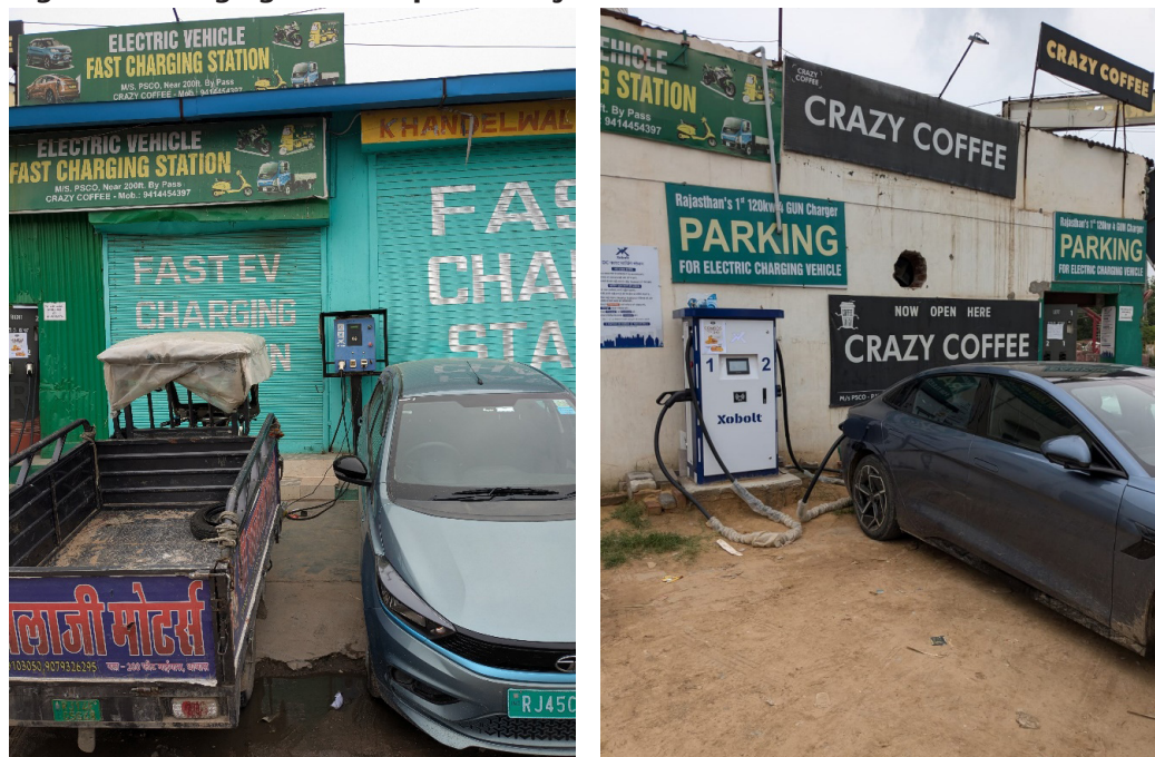
Figure 6: Charging station operated by XoBolt
