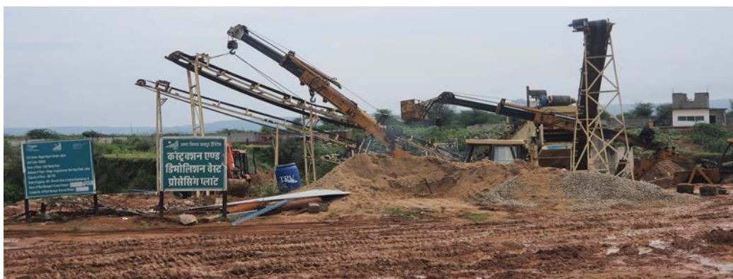
C&D waste processing plant in Langariyawas, Jaipur
