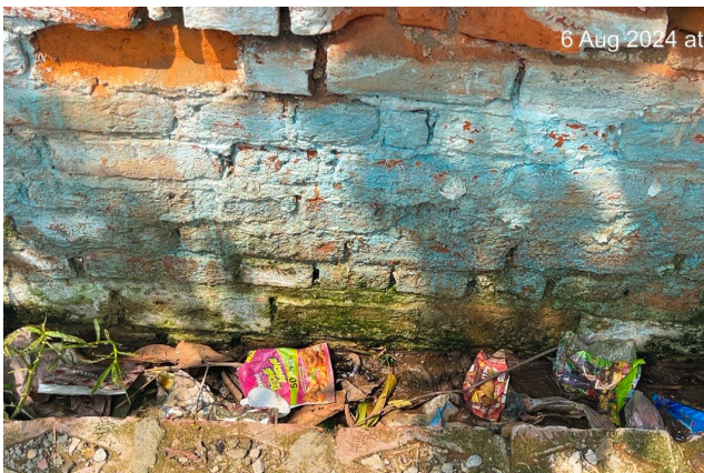
Drains are blocked with solid waste, which makes them non-functional for grey water to flow through in Bhandpura village.
