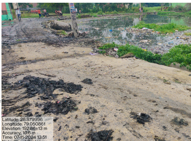
Drains open directly into the village pond, causing them to overflow during the rainy season in Khaul village, Saidnagar block.
