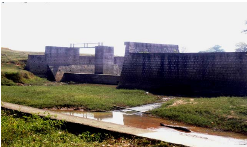
Figure 5 : Check dam at Ormanjhi block, Ranchi (Government's Water Supply plant) as a part of field exposure with Hazaribagh's participants
