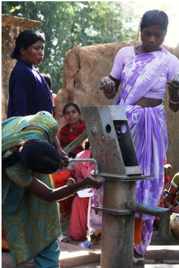
Figure 3: Hand pump mechanics repairing a hand pump in Mander block, Ranchi with participants from Khunti
