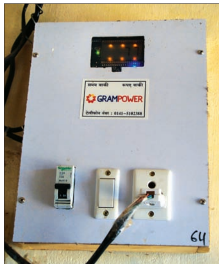
Micro-grid technology provider Gram Power has installed prepaid smart metres in Pali district, Rajasthan
