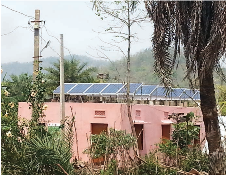
A view of the solar mini-grid in Rajanga Village in Odisha
