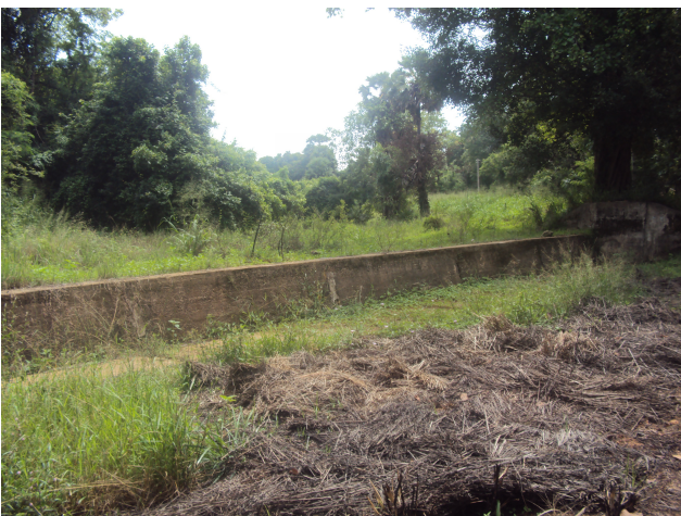
Photograph 8: Sluice for tackling runoff from Periakulam wewa to Pudukulam wewa in Anuradhapura district. Source: Sushmita Sengupta, Water Team, CSE
