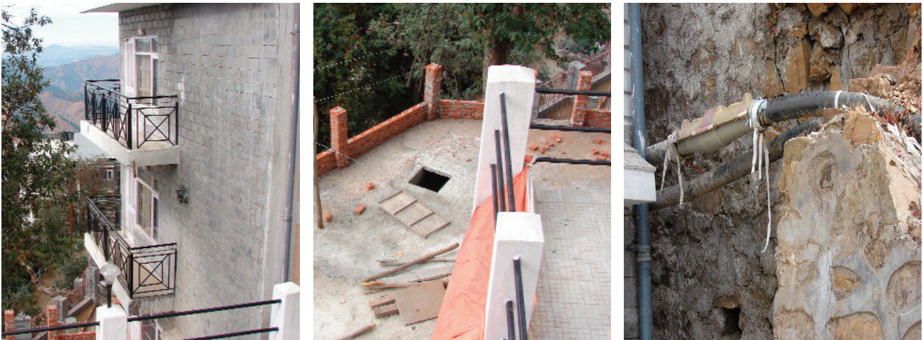
Picture 5 Nirmal Awas Residential Apartments (a) Nanak Kutti Residential apartments (b) A septic tank under construction (c) Broken sewage pipes
