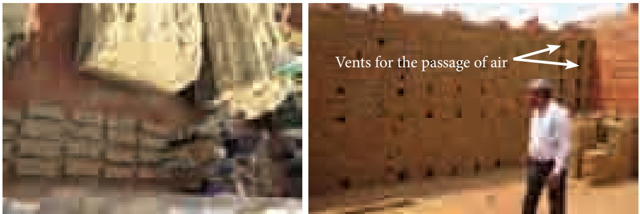
Figure 24: Brick setting in chambers in an induced zigzag kiln
