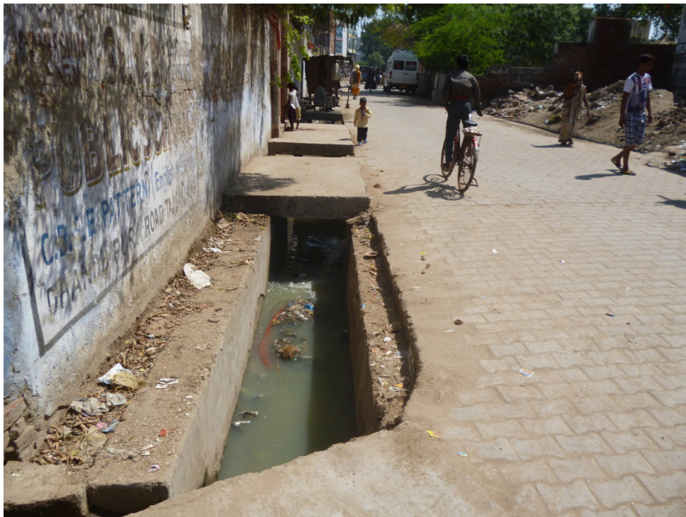
Figure 8: Open drain in the city (Source: Shantanu/CSE, 2015)
