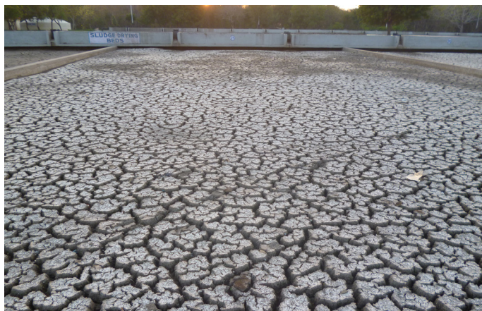
Figure 2: Sludge drying bed - UASB technology 78 MLD STP in Dhandupura (Source: Rahul/CSE, 2015)
