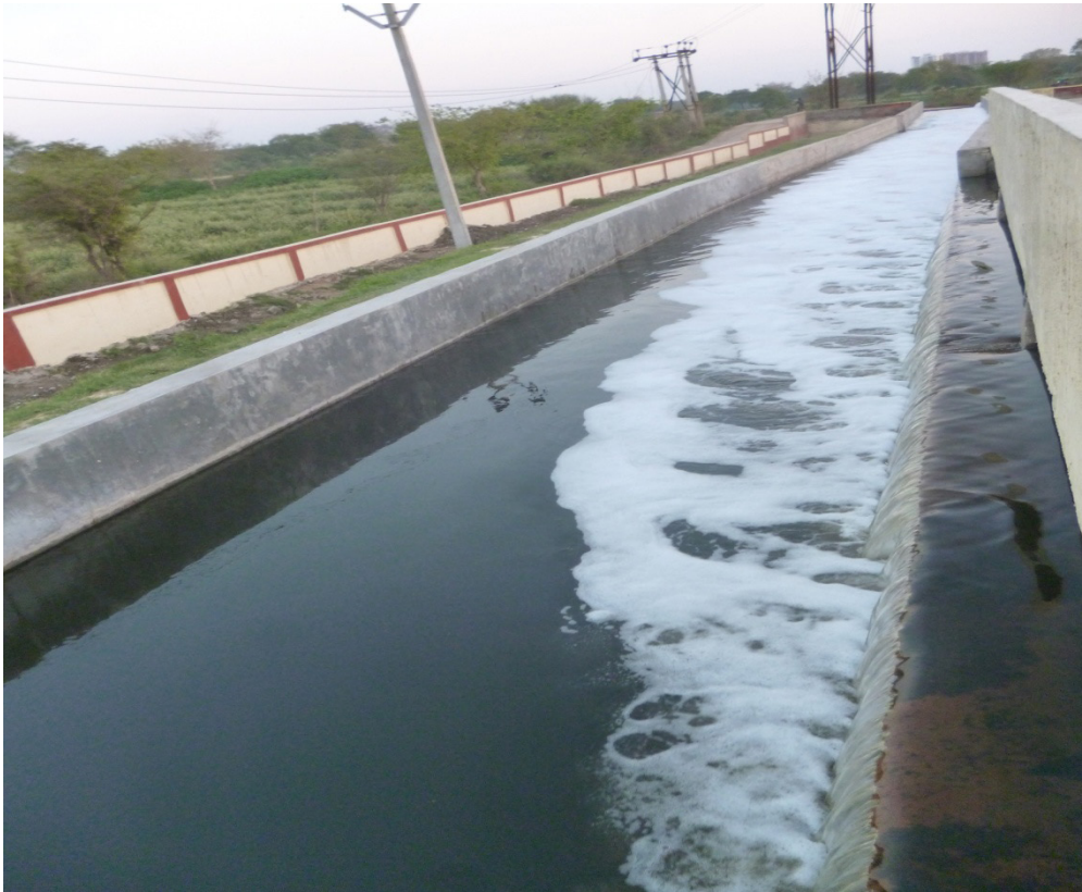
Figure 7: Outfall of Dhandupura STP (Source: Shantanu/CSE, 2015)
