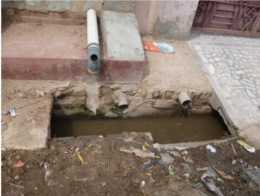
Figure 3: Night soil disposed into open drain (Source: Shantanu & Rahul/CSE, 2015)
