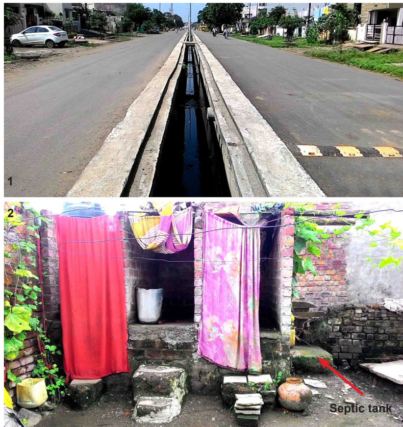
Figure 5: Trunk sewer and containment system (Source: Shantanu/CSE, 2015)
