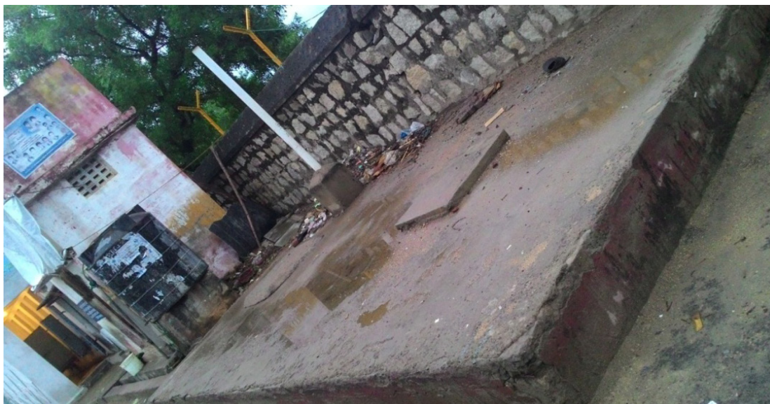
Figure 2: Septic tank connected to community toilet in Ariamangalam slum (Source: Bhitush/CSE, 2015)
