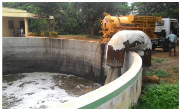
Figure 4: Septic tank connected to community toilet in Ariamangalam slum (Source: Bhitush/CSE, 2015)
