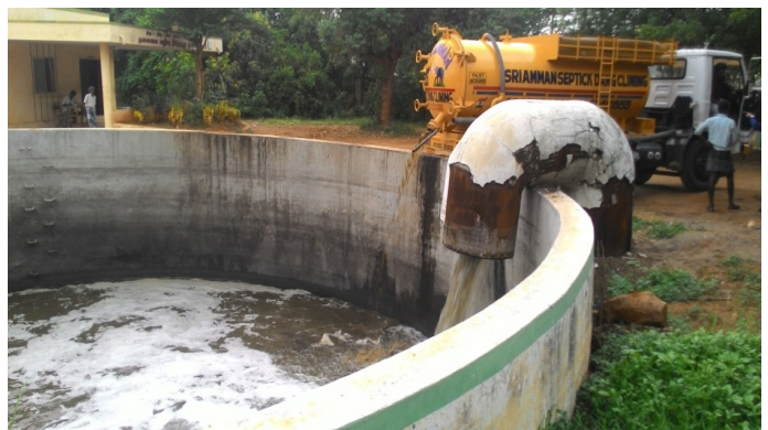
Figure 2: Septic tank connected to community toilet in Ariamangalam slum (Source: Bhitush/CSE, 2015)
